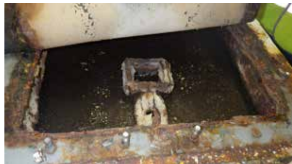
Sewage treatment plant defective
