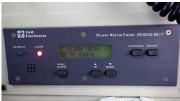
MF-HF radio power alarm
