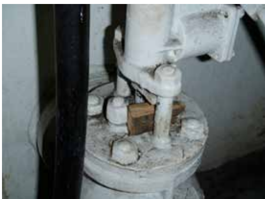
Service tank valve secured open
