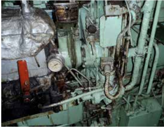
Diesel generator insulation saturated with oil
