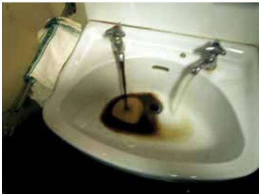
Dirty hot water supply
