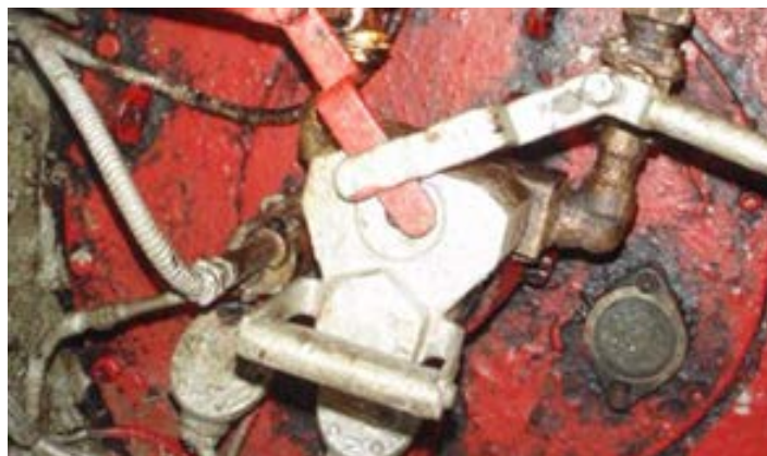
Figure 2: Missing screening of boiler fuel piping connections
