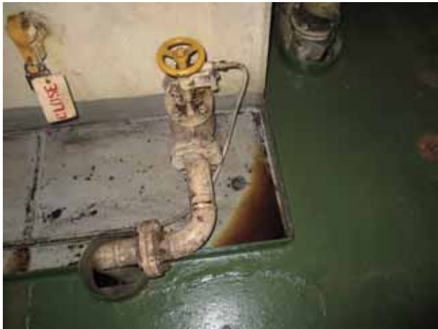
Oil leakage and accumulation
