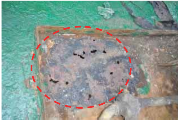
Corrosion holes on strength deck
