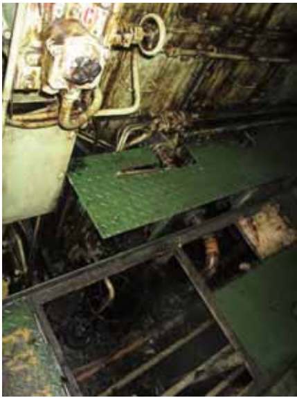
Oily and dirty engine room
