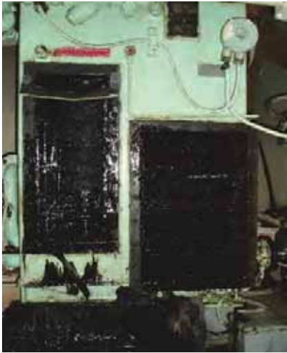
Clogged oil water separator
