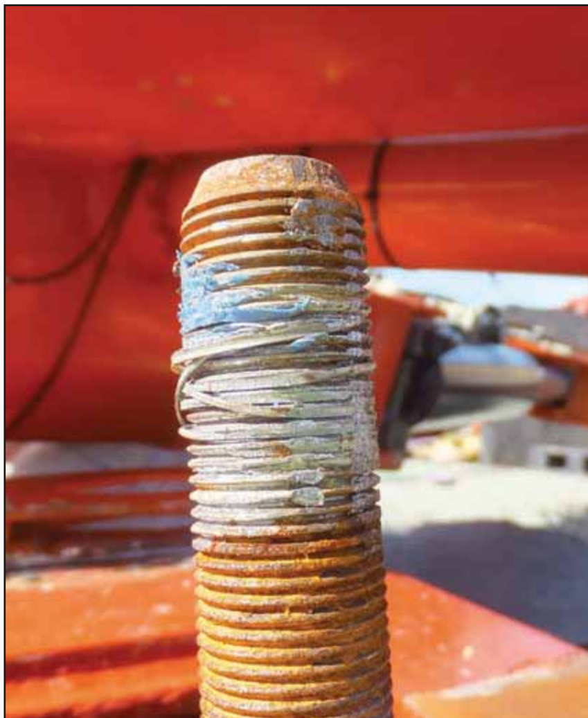
Figures 2 and 3: Failed nut and tie bolt
