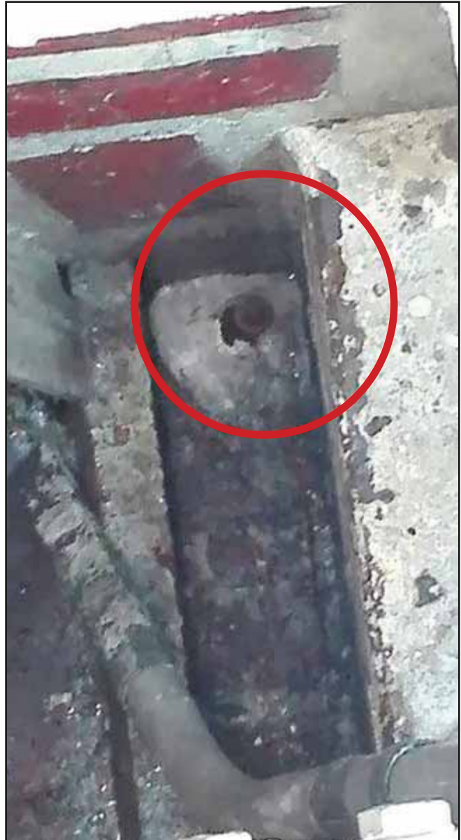
Figure 3: Bung in place
