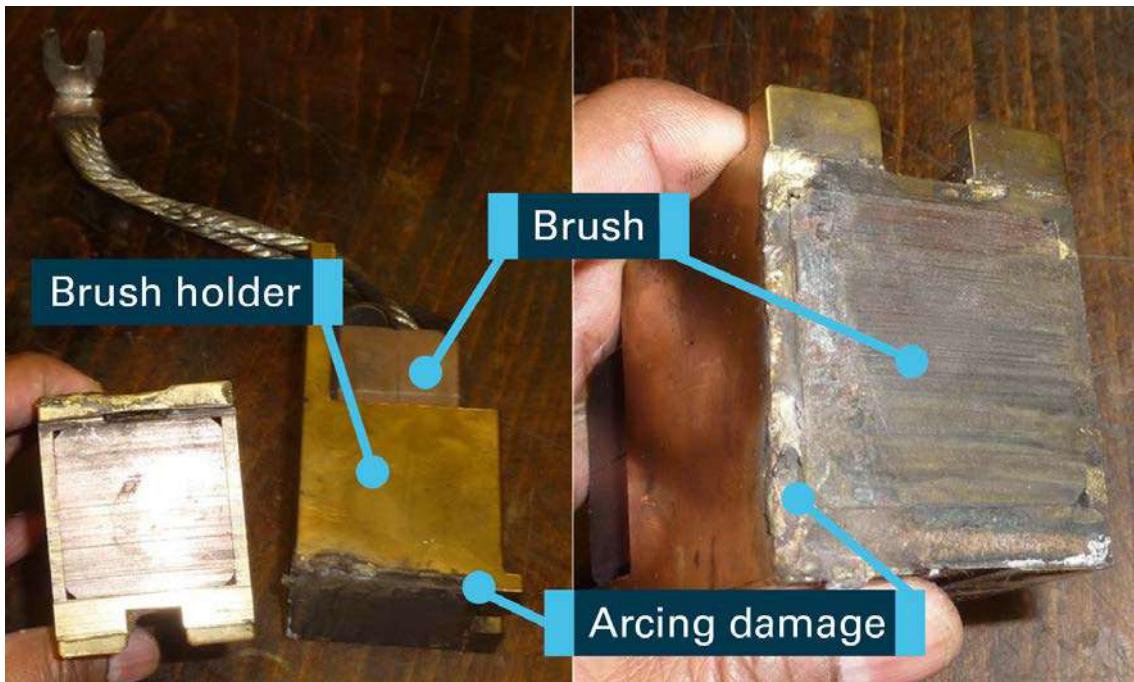
Figure 7: Arcing damage to brush holders
