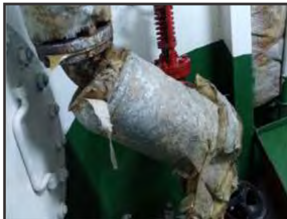
Insulation arrangement from emergency fire pump inlet pipe wasted
