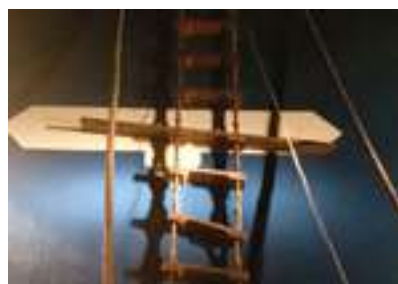
Figure 11 – The step on this ladder gave way whilst the Pilot was disembarking
