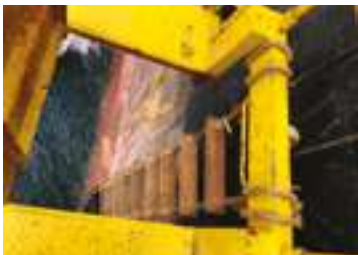
Figure 7 – Ladder does not extend 1.5 metres above the trap door – how do you transit from ladder through the trap door?
