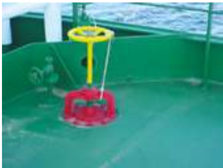
Figure 3 – Deck oil spill dump valve
