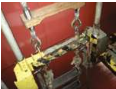
Figure 8 – Two stage non-compliant ladder – weight is not held by man ropes at all
