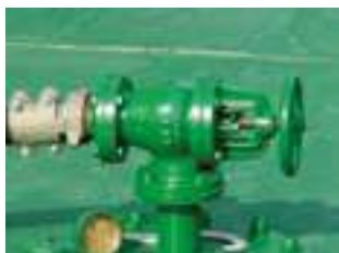
Figure 5 – Wilden pump discharge connection to slop tank
