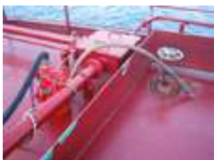
Figure 4 – Aft end Wilden pumping arrangement
