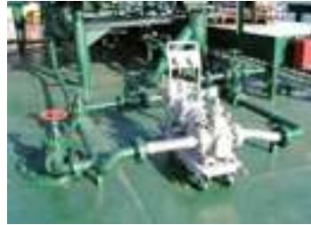
Figure 6 – Midship pumping arrangement at manifold
