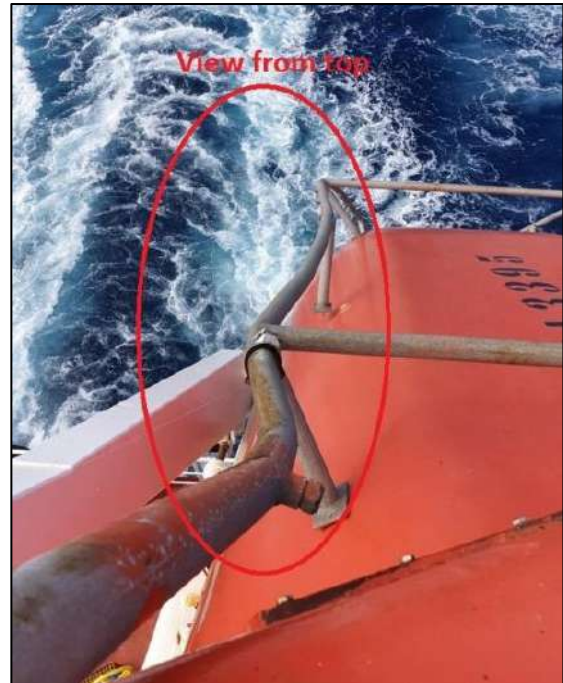
Figure 3: Damage to lifeboat's sprinkler system
