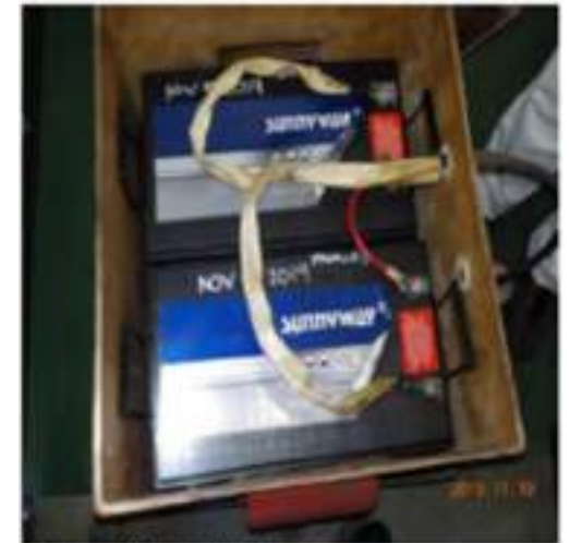
New GMDSS batteries
