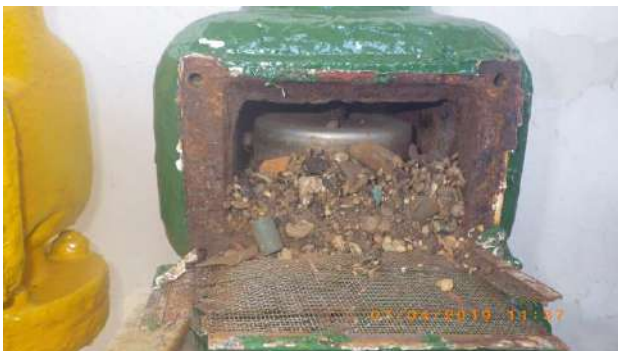
Candidate photo for Deficiency Photo of the Year
