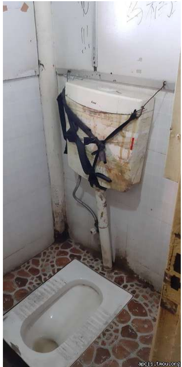
Candidate photo for Deficiency Photo of the Year
