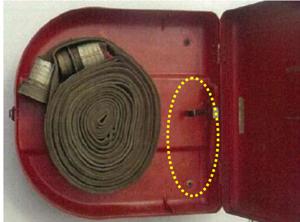
Hose nozzle missing.
