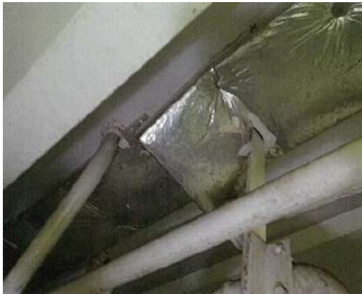
Deteriorated insulation on underside of deck.
