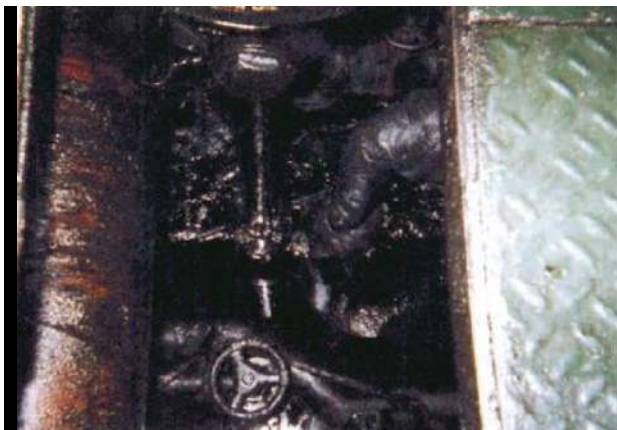
Tank top of engine room oily.
