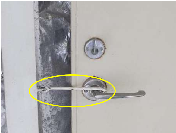
Unacceptable hold-back hook.
