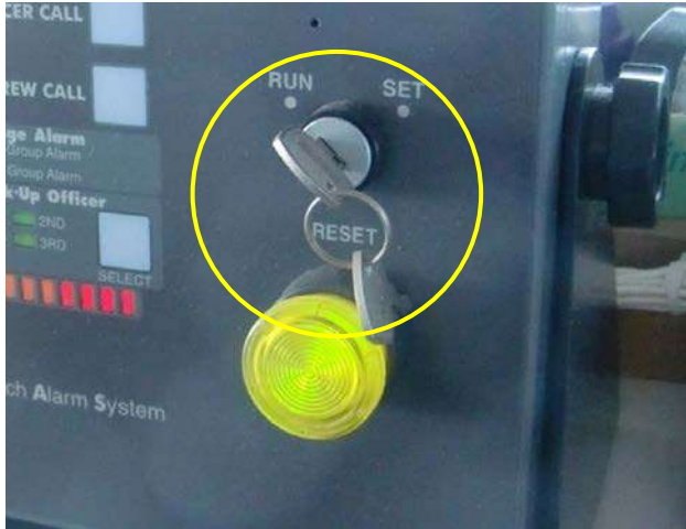
Keys left in BNWAS control board. (Not properly secured.)
