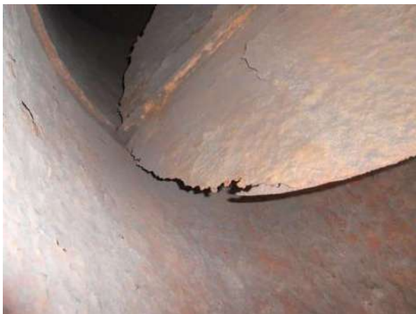
Fire damper flap wasted.
