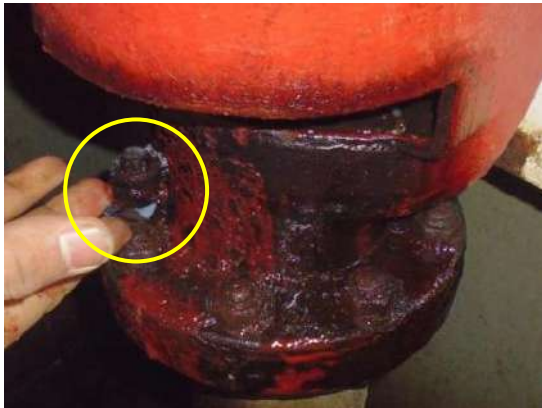
Bolt unfastened and air pipe head leaking oil.
