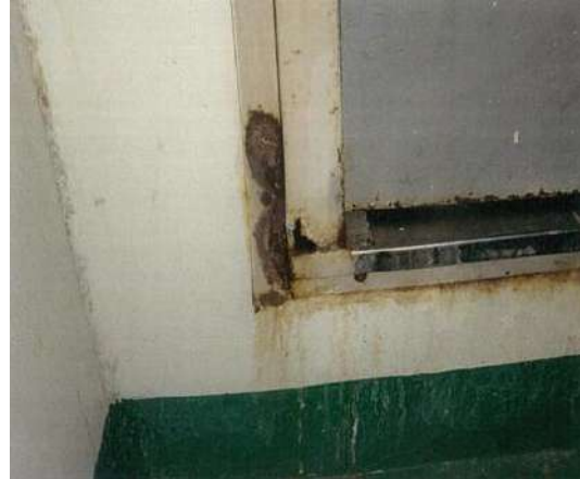
Worn-out and partially wasted fire door frame.
