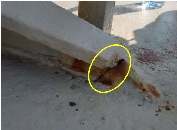
Cracked hatch coaming end bracket.
