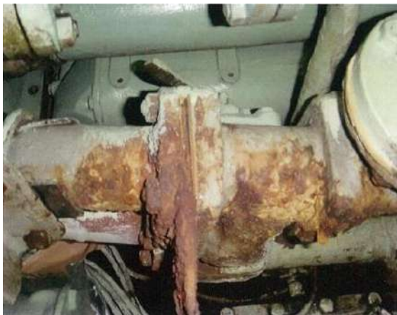
Badly corroded and leaking piping.
