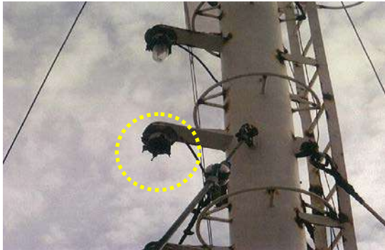
Signal light missing.
