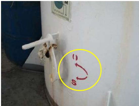
"Open-shut" positions clearly marked on ventilation trunk.
