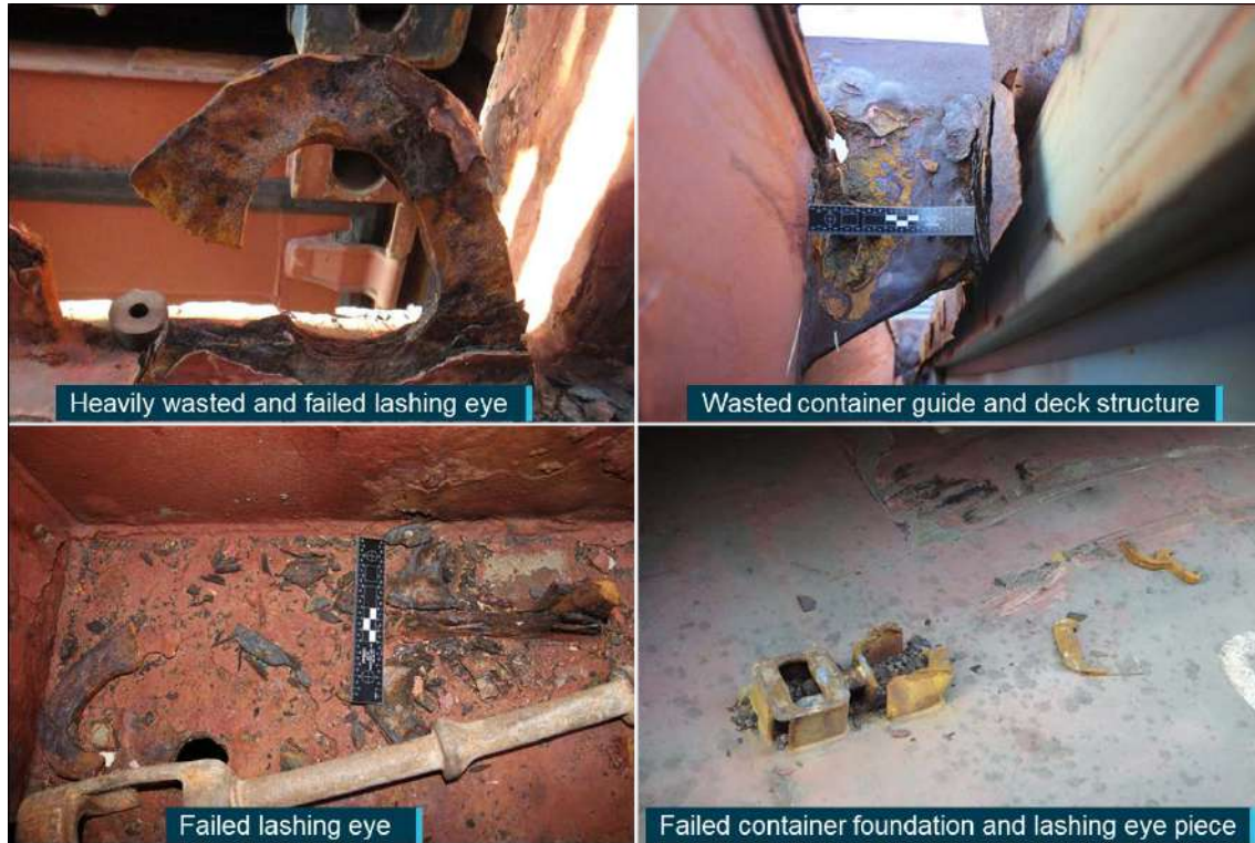
Figure 4: Examples of condition of cargo securings and ship structure
