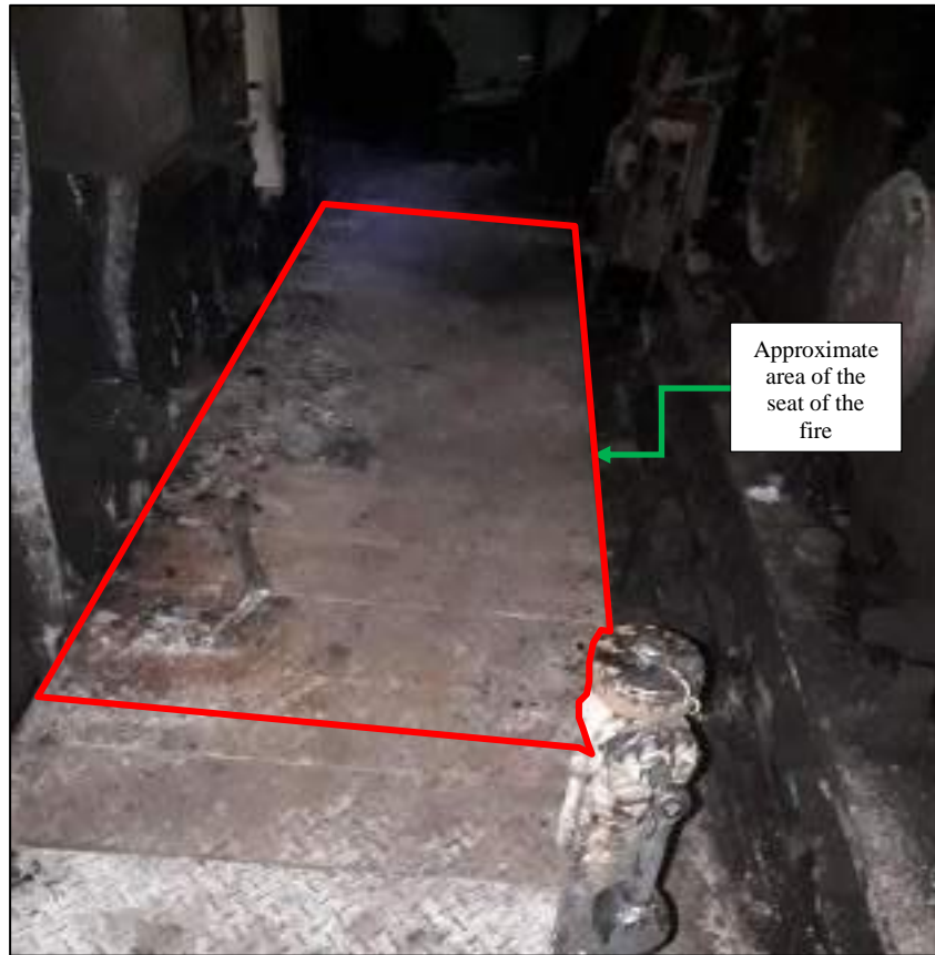
Figure 11: Seat of the fire on the main floor in the propulsion room
