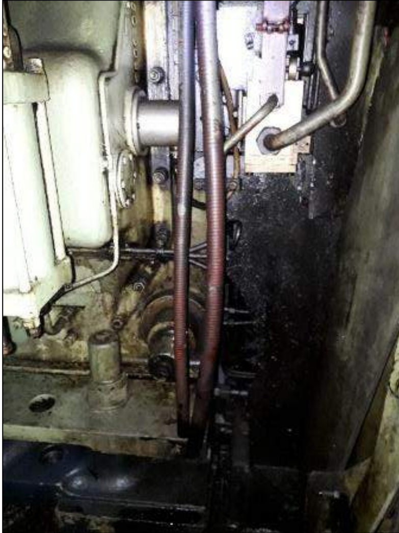
Figure 12: PVC braided pipes used to direct leaking oil from the port engine
