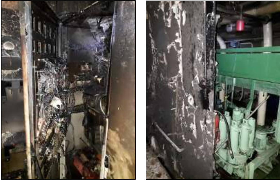
Figure 7: Burnt out electrical / control panel forward of the ECR and modules room bulkhead
