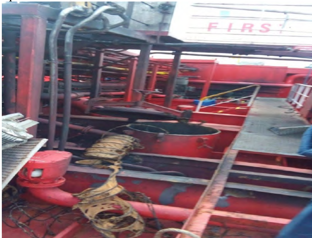
A fixed gas freeing fan and venting line is fitted on deck. The flexible venting tubes are connected to the venting line.
