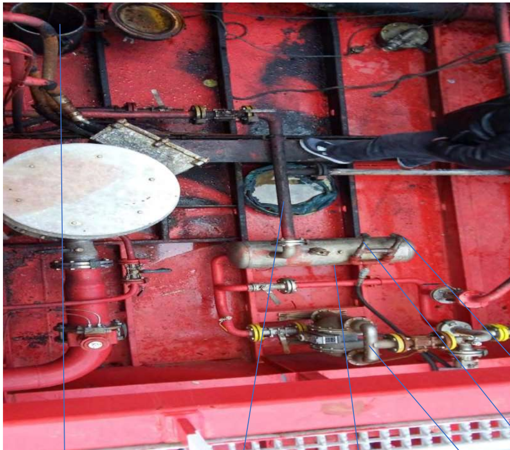
Sounding /Sighting Port Pipes
