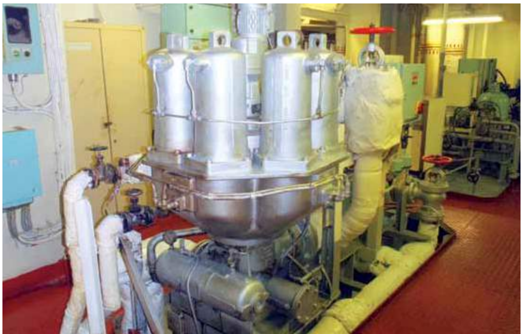
^ Fuel oil filters
