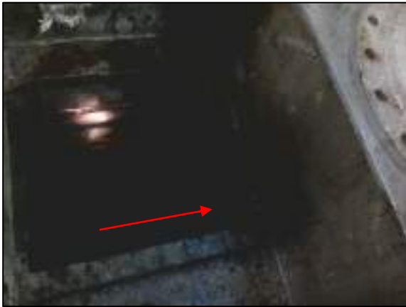
Figure 7: Access manhole opened (red arrow indicates direction towards starboard side bilge alarm sensor, through a lightening hole)
