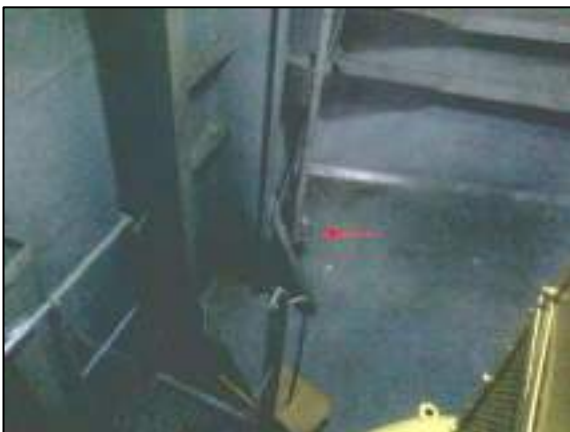
Figure 4: Port side bilge alarm sensor (red arrow), as seen from the lowest pump room gratings
