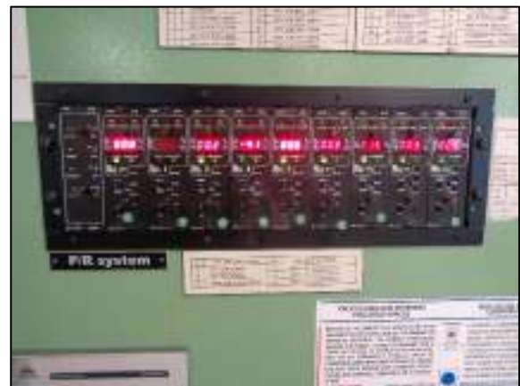
Figure 11: Display panel of the fixed gas detections system
