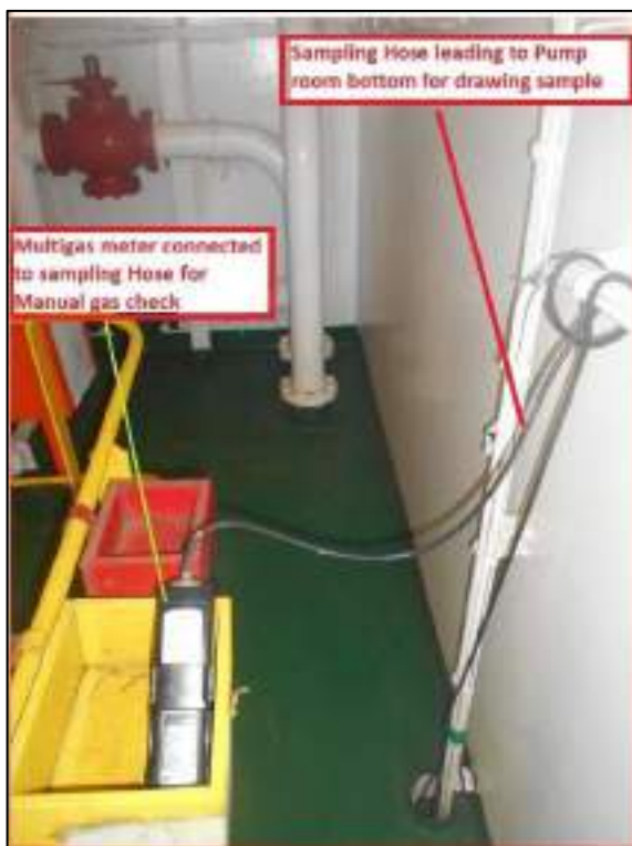
Figure 12: Personal multi gas detector placed at the pump room's entrance
