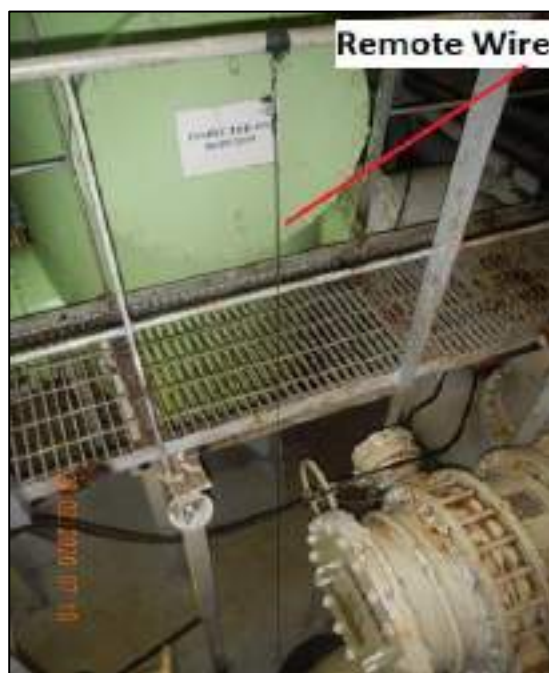
Figure 17: Wire to remotely test the starboard bilge alarm
