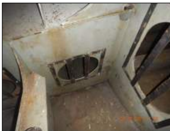
Figure 18: Lightening holes within the starboard bilge space blocked
