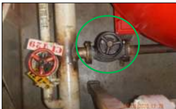
Figure 15: Suction valve (circled in green) of the starboard bilge of the pump room
