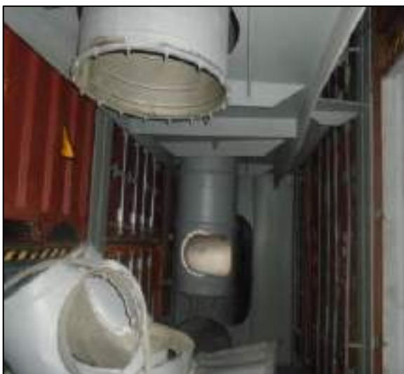
Figure 4: Mechanical ventilation duct damaged
