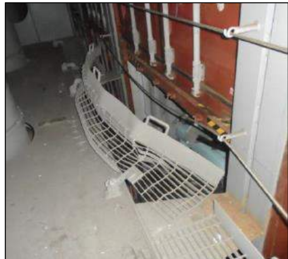
Figure 5: Distortion of steel walkway platform
