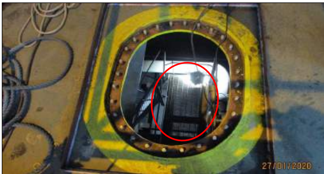
Figure 8: Access to WBT no. 1006 - First level platform with lighting installed marked
