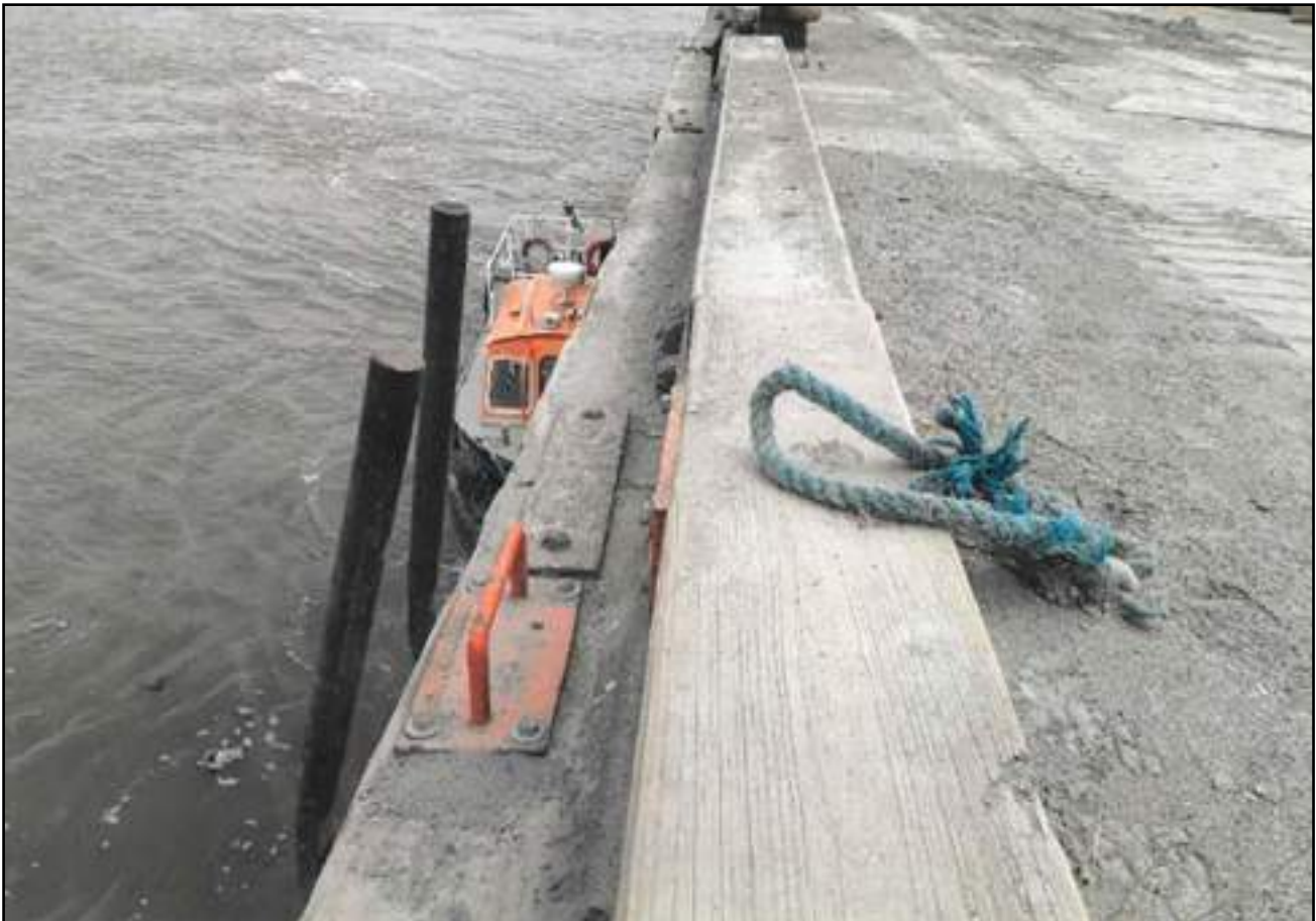
Figure 3: Quayside showing ladder and loose aggregate
