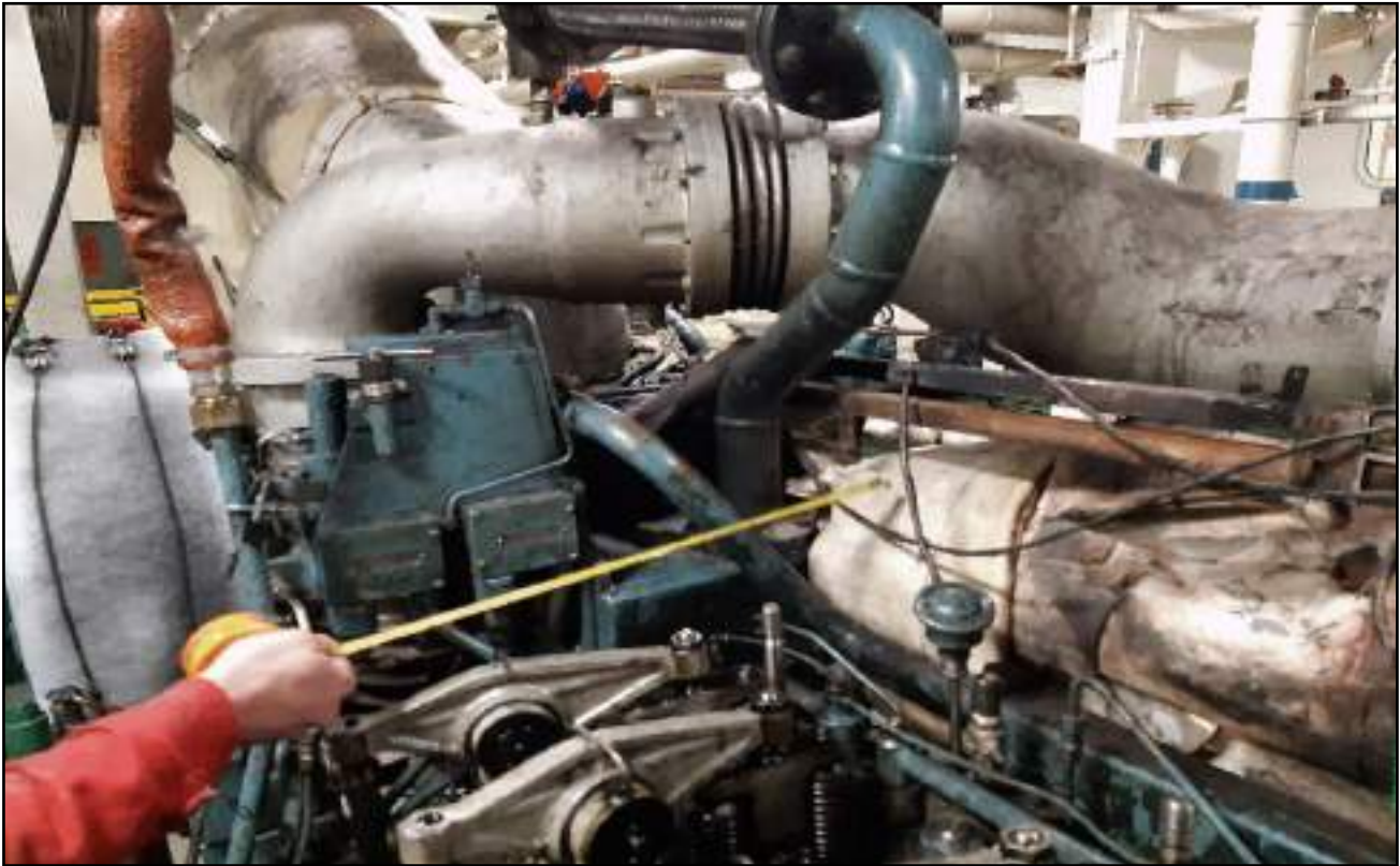
Figure: Location of lagging that ignited indicated
