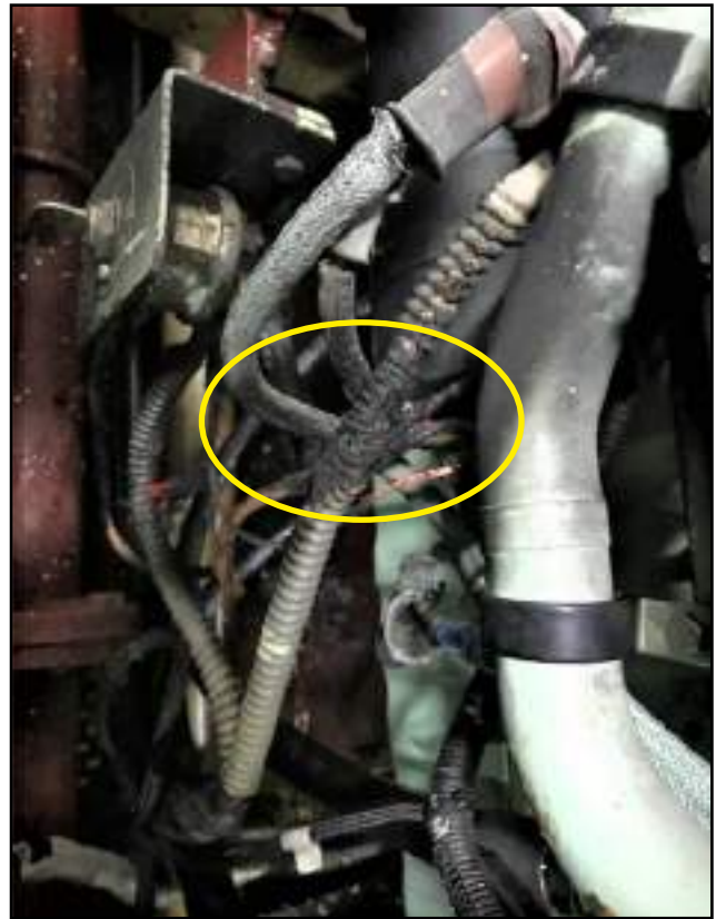
Figure: Heat damaged electrical cabling
