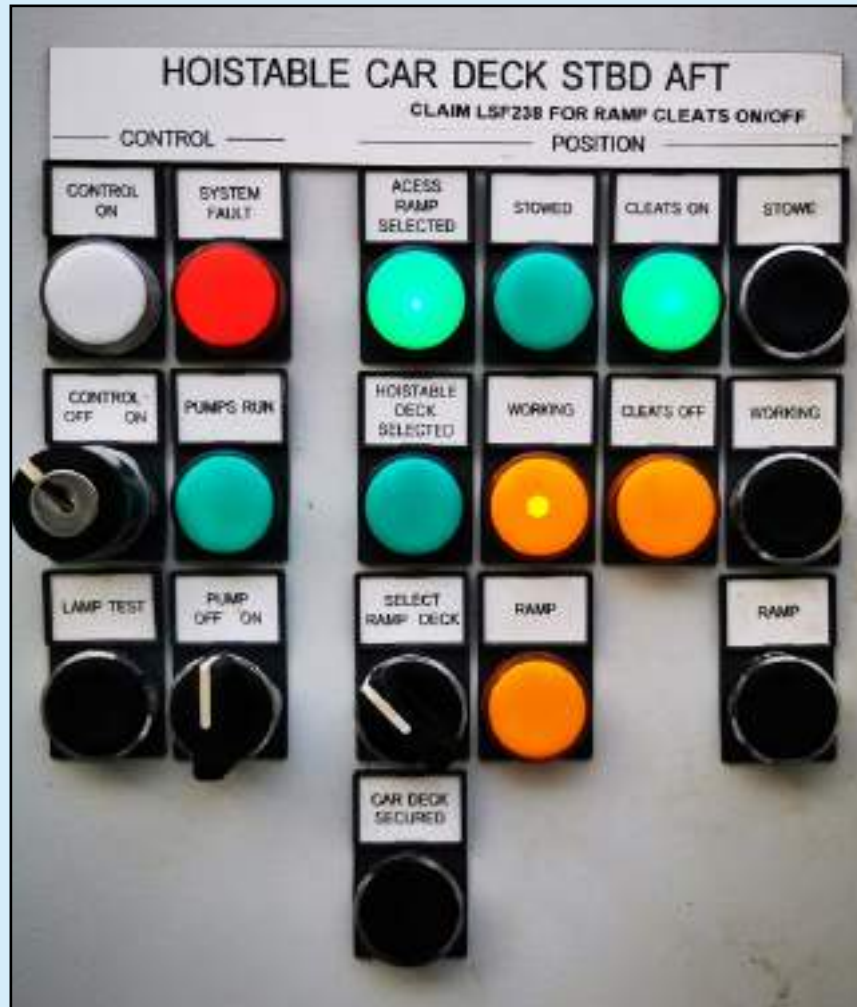
Figure 2: The hoistable car deck control panel
