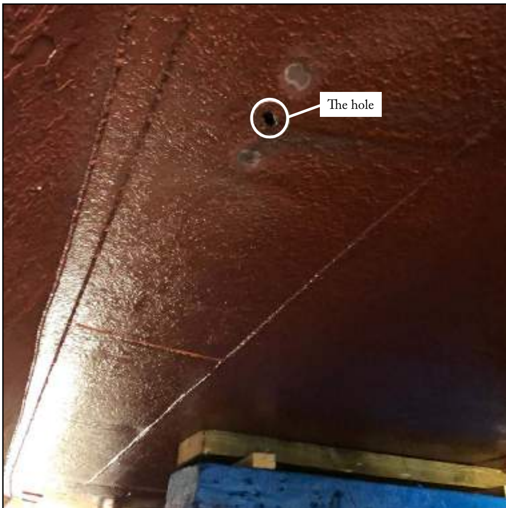
Figure: The 25mm hole in the fishing vessel's shell plating, observed when the vessel was lifted out of the water.
