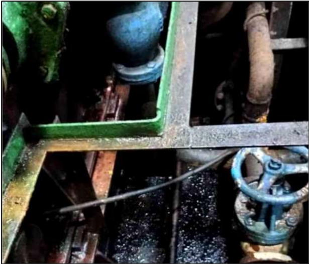
Dirty condition in engine room
