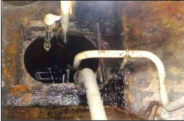
Dirty condition in engine room
