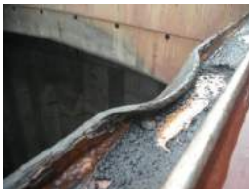
Figure 2: Damaged cargo hatch sill
