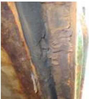
Figure 5: Hardened indented rubber seals
