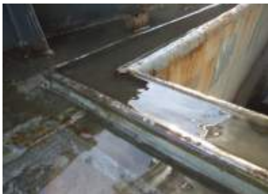
Figure 3: Overflowing drainage channels
