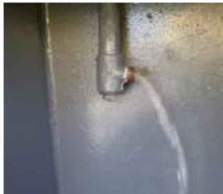
Figure 4: Non-return valve not fitted to the drainage arrangement
