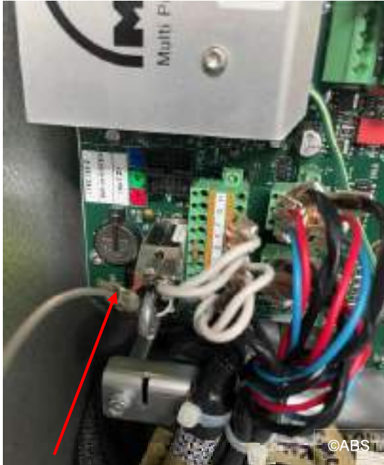
Main engine battery replaced in Engine Control Unit
