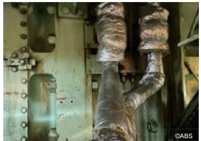
Fuel piping found without insulation – after
