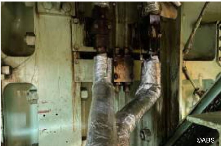
Fuel piping found without insulation - before
