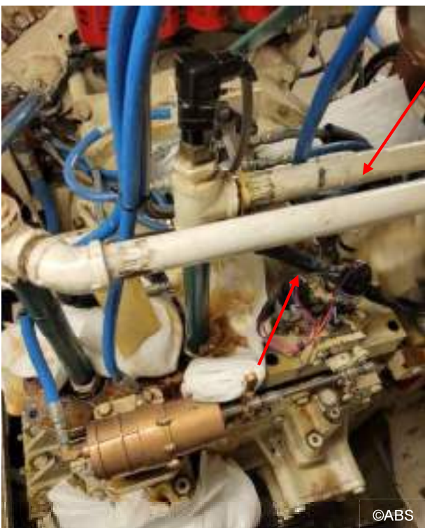
Main engine fire due to a cracked lube oil pipe fittings – before
