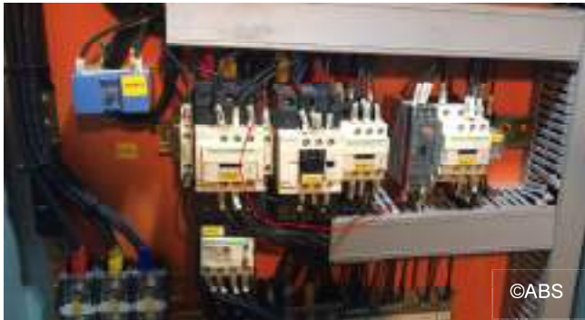
Emergency fire pump defective controller replaced
