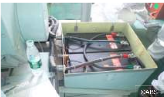
Emergency generator would not start; new batteries installed
