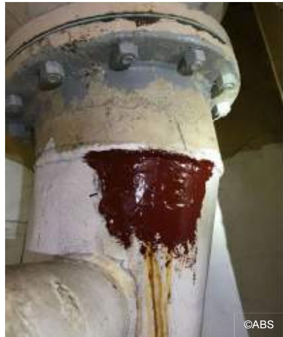
Ballast piping found with soft patch
