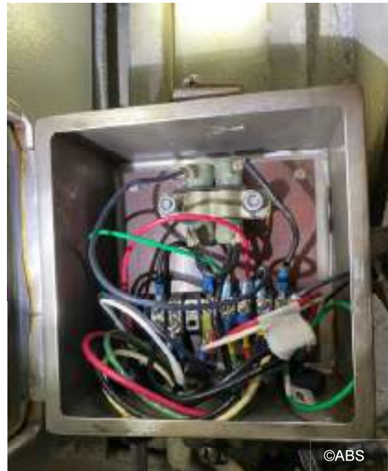
Bad connection from the transformer voltage to the power relay in the steering gear control box repaired
