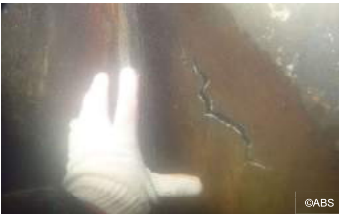
Owners are to report all damages that may affect classification. Side shell found damaged outside - before
