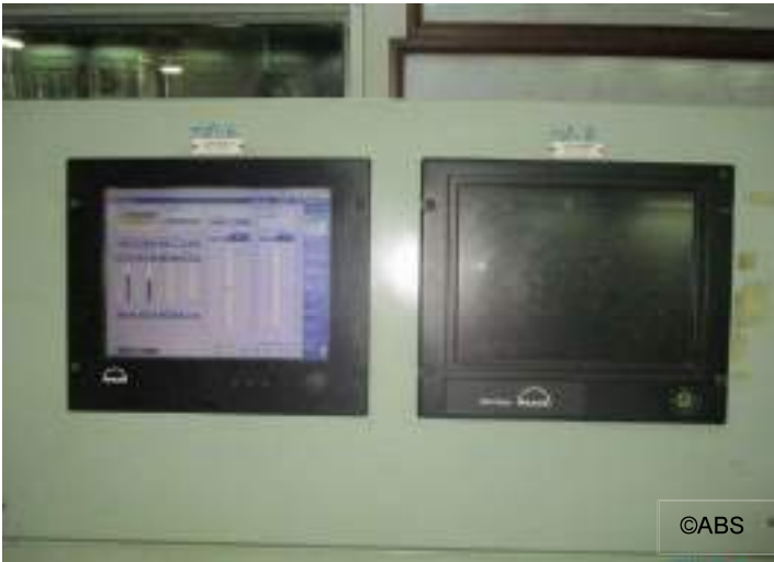
Main engine defective component for CPU replaced
