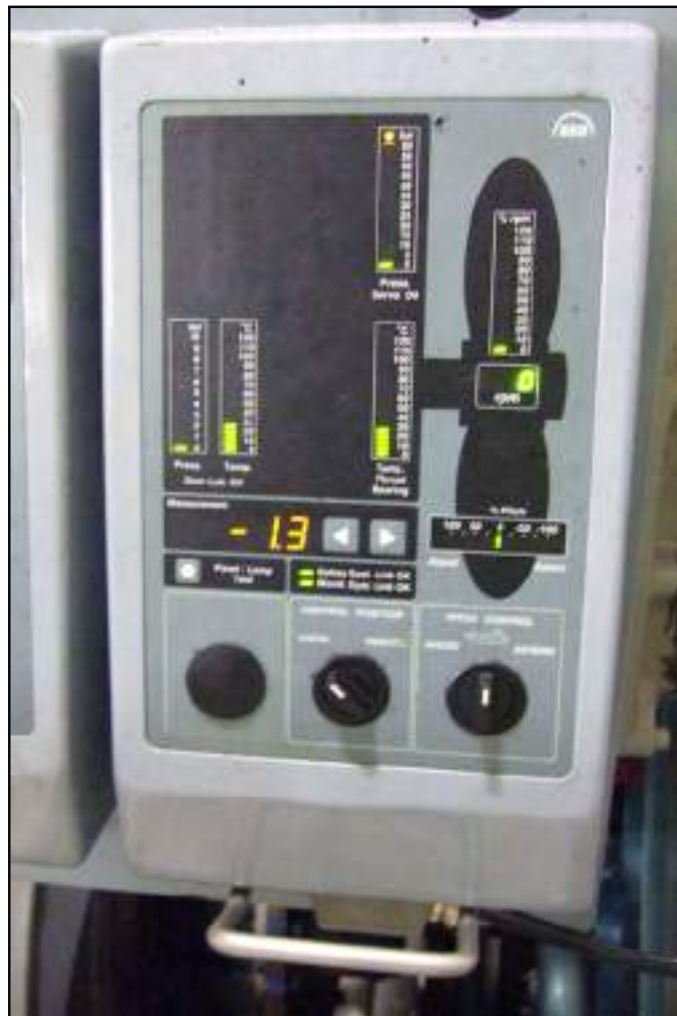
Figure 8: Local control for main propulsion system
