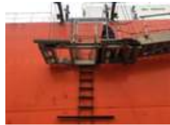
Non-compliant trapdoor arrangement.
