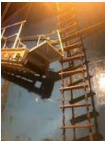
A non-compliant combination arrangement.
