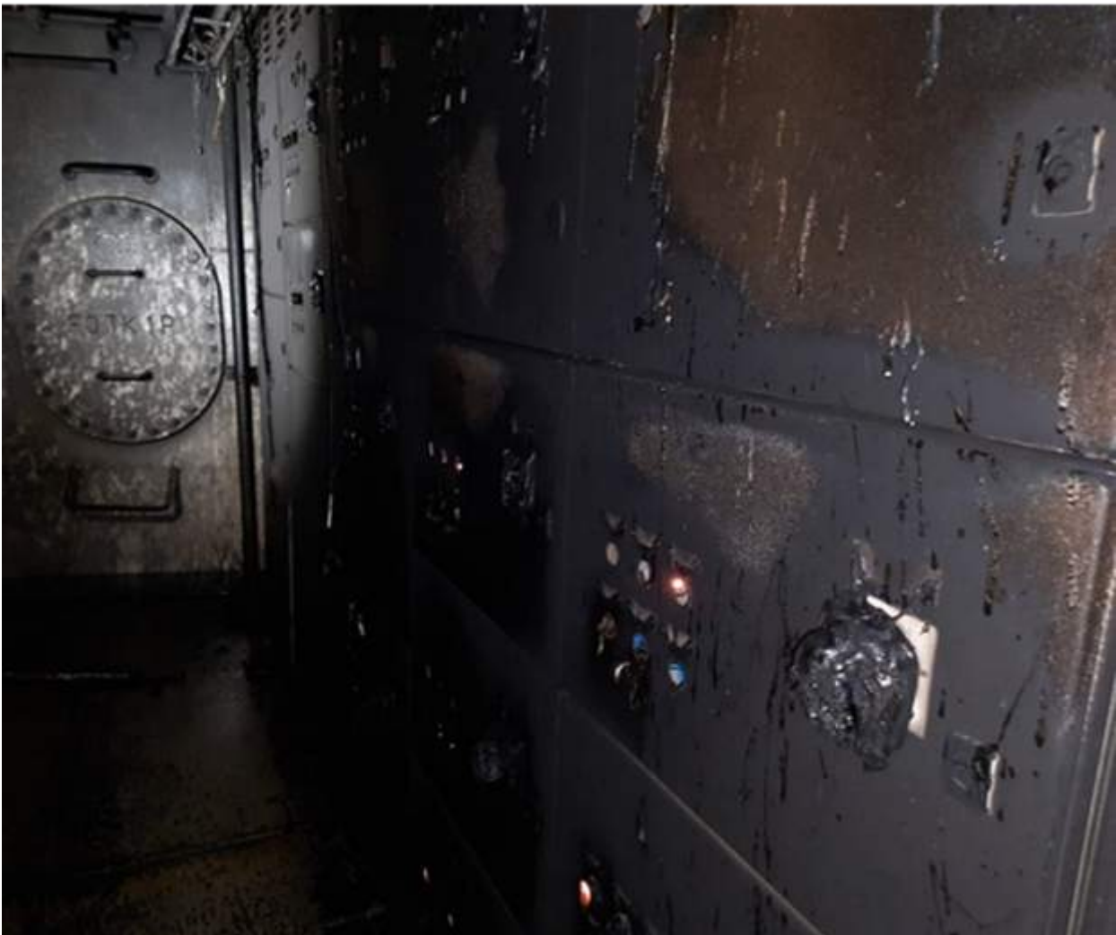
Figure 6: Fire damage inside the port engine room
