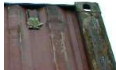
Figure 5.20 Vent tapped over
