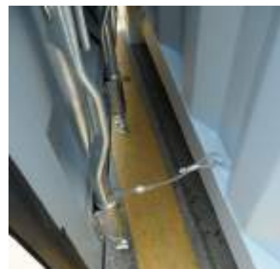
Figure 5.30 Door retaining strap
