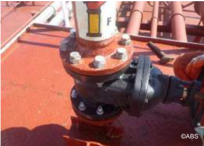
Foam station valve found with broken valve casing replaced
