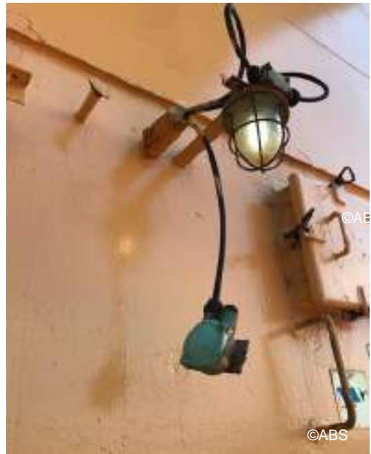
Damage to electrical installations
