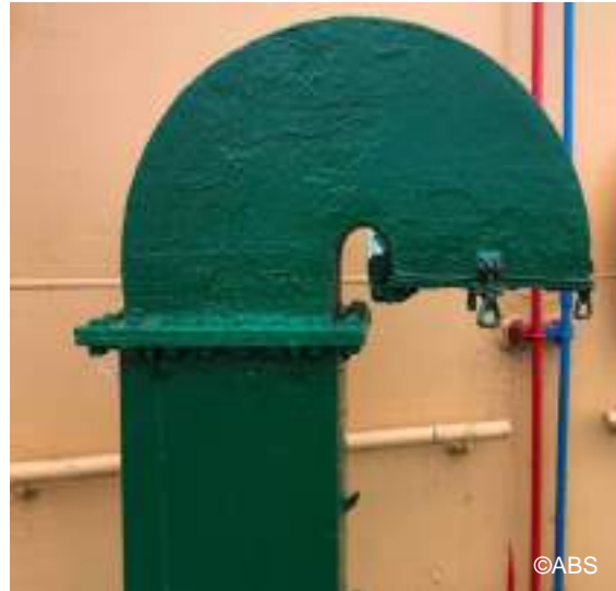
Ventilator found corroded – after
