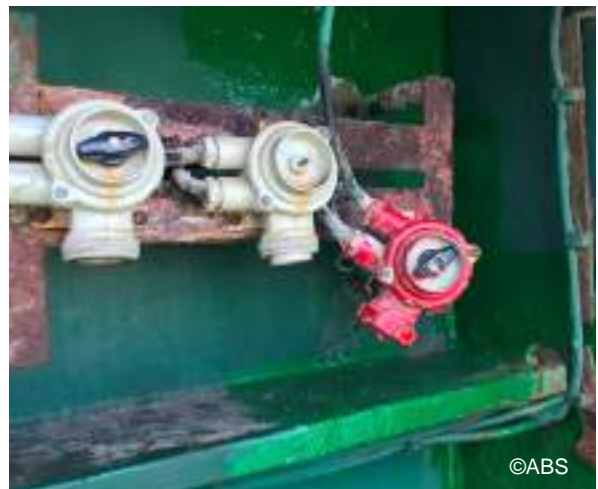
Damage to electrical installations
