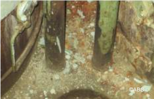
Main engine cylinder cooling water leak
