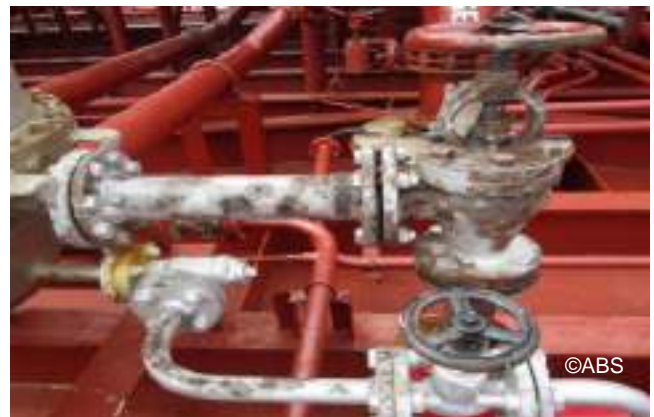
Steam pipe found with corrosion
