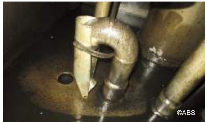
Funnel area – oil spillage from tank airpipe
