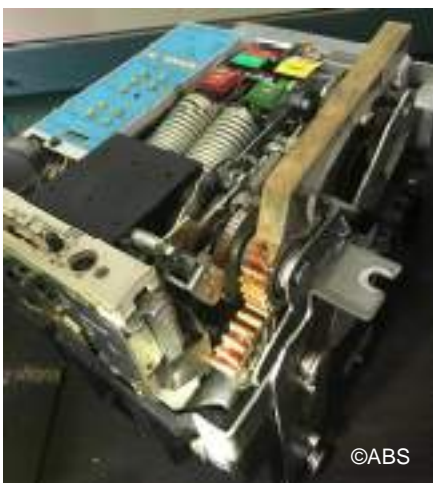
Emergency switchboard air circuit breaker damaged
