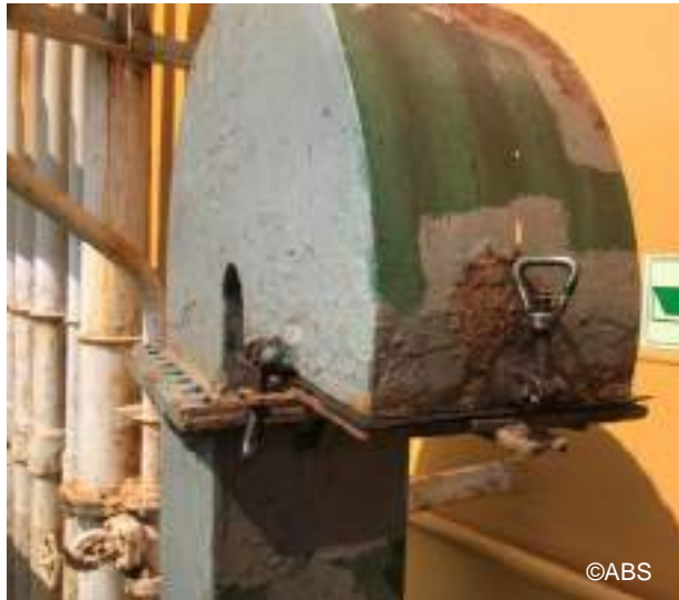
Ventilator found corroded - before
