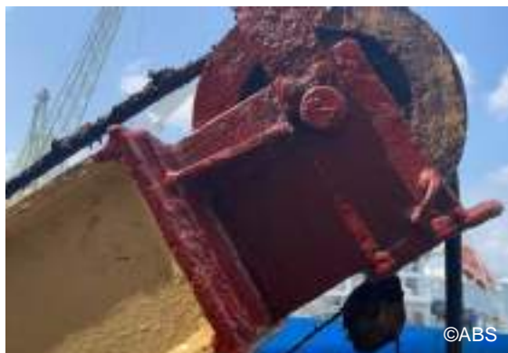
Rescue boat davit found corroded
