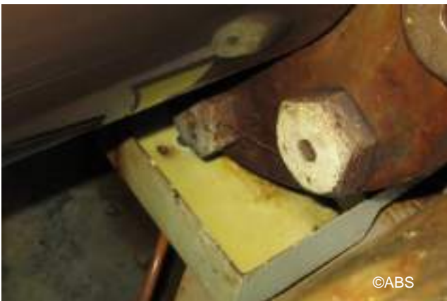
Steering gear leaking oil
