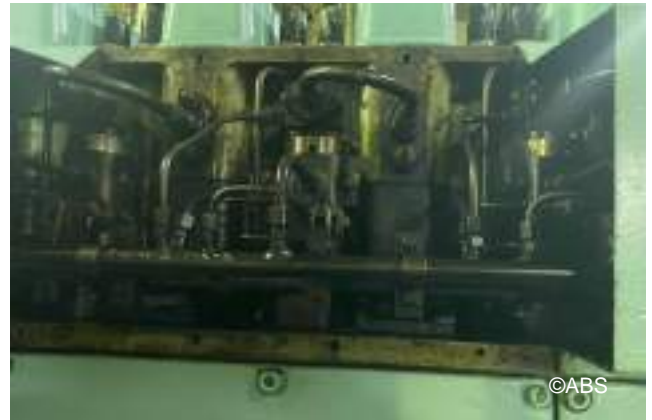
Main engine fuel pump leak
