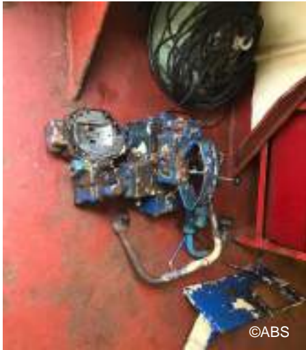
Damaged hydraulic motor for mooring winch removed
