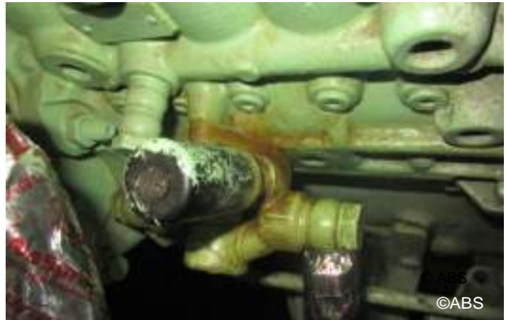
Emergency diesel generator high pressure pipe leak
