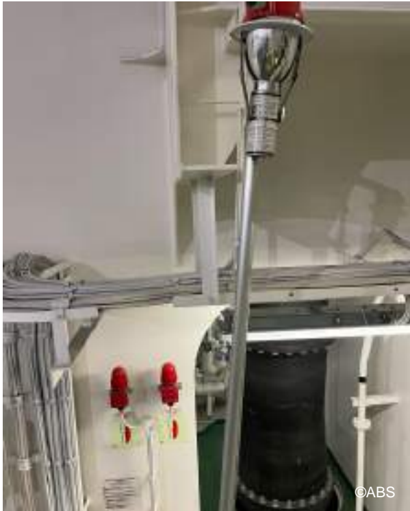
Testing engine room fire detector after repair
