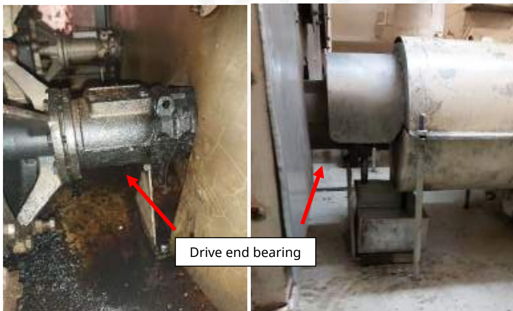
Spray guard position in relation to drive end bearing Pride of Hull (left) and Pride of Rotterdam
