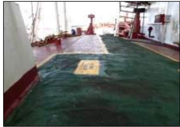
Figure 4: Bulging of the open deck, directly above FOT no. 2P
