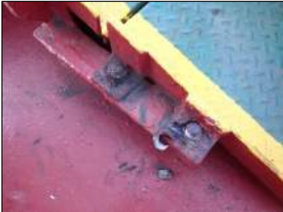
Figure 10: One nut had been successfully cut by the angle grinder, before the explosion occurred
