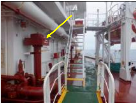
Figure 8: The vent head of FOT no. 2P against the accommodation block on port side
