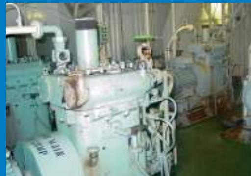
► Typical air compressors on a vessel
