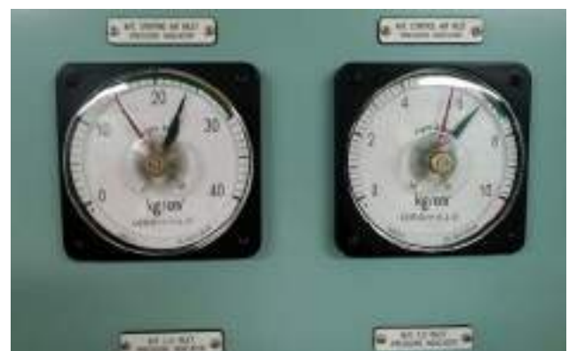
Good start air pressure with safe operational limits marked
