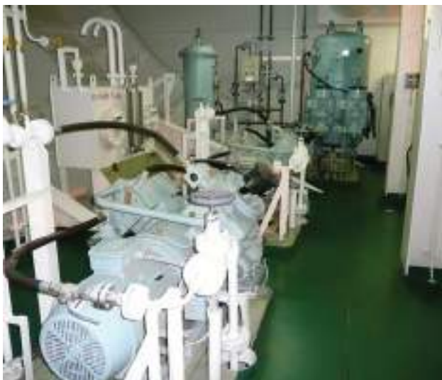
Main air compressor
