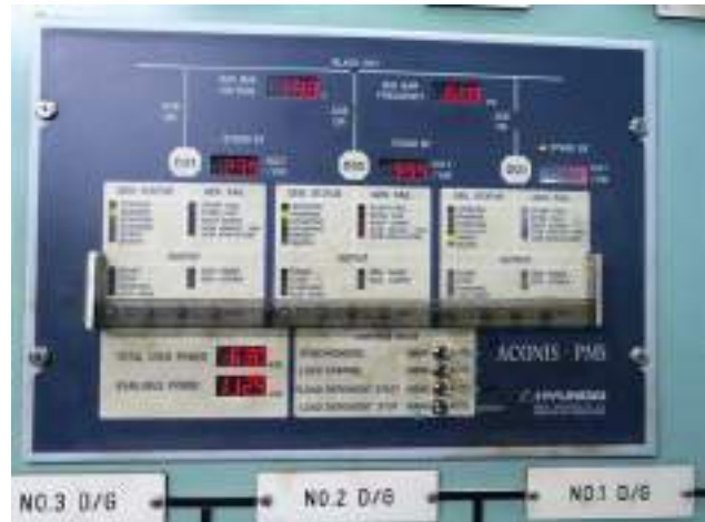
Switchboard load out of balance
