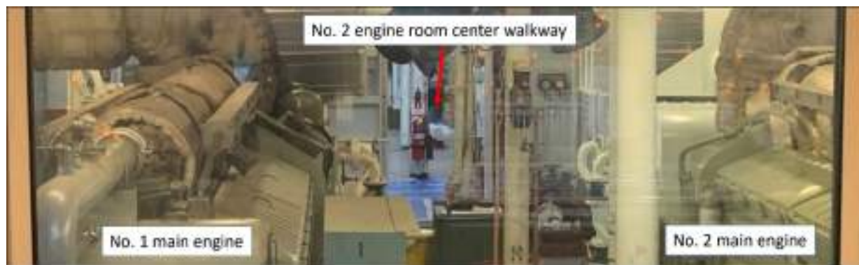
Figure 4. No. 1 engine room diesel engines as seen from the EOS; center walkway of the no. 2 engine room is through the open door in the background. (Source: WSF)
