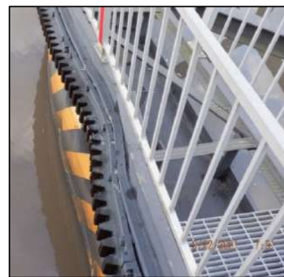
Figure 5. Damaged steel plating and rack on gate.
