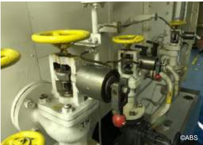
Lubrication oil system quick closing valve inoperative
