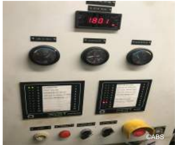
Crew not familiar with procedure to manually connect emergency generator to switchboard
