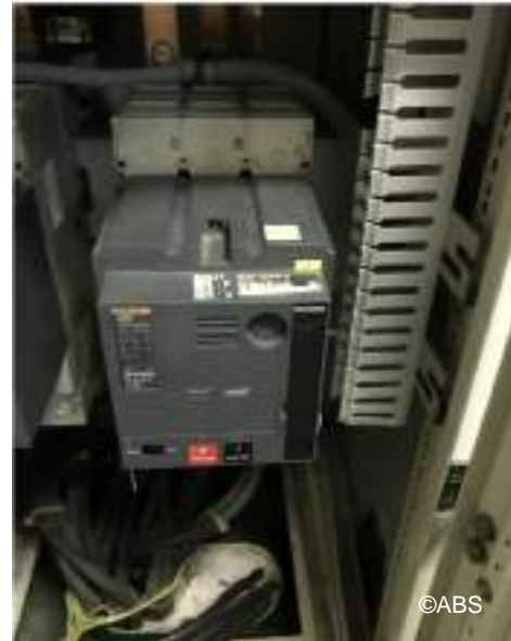
Automatic Voltage Regulator (AVR) of emergency generator malfunctioning
