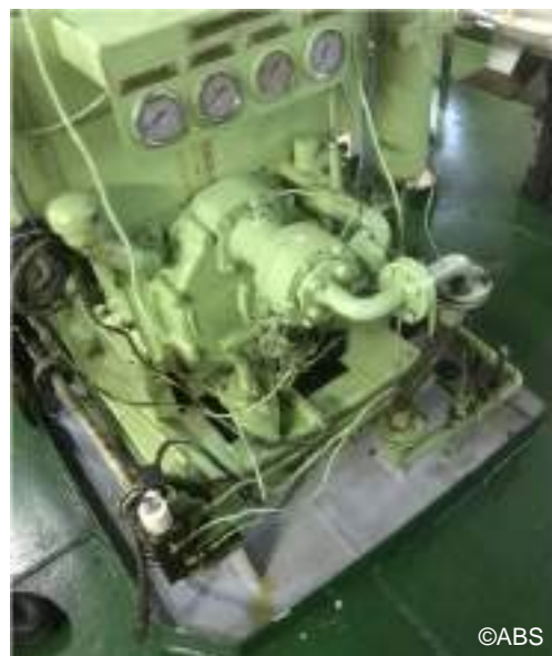
Oil leakage from main air compressor pumps
