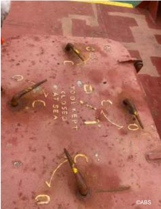
Cargo holds entrance unable to close due to worn handle, turning to 360 degrees on actual closing
