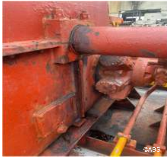
Oil leakage from winches on deck
