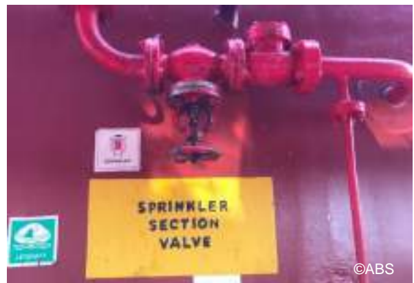
Paint room sprinkler system not in operation due to isolation valve stuck
