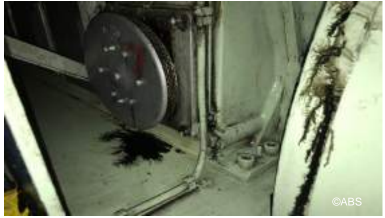
Oil leakage from generator engine crank case explosion door and fly wheel end seal
