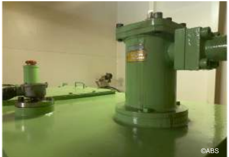
Leakage of deck machinery hydraulic pump circulating system located at Forecastle Space
