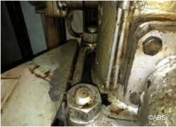
Oil leakage from main engine fuel pump
