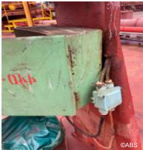
Unsecured junction boxes and cables on deck
