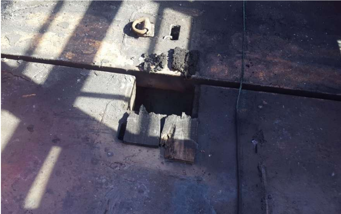
Figure 2: Tween deck gaps
