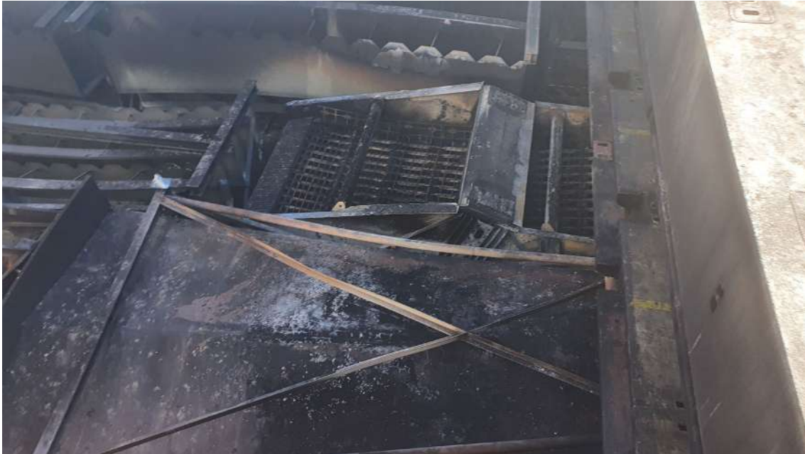
Figure 5: Burnt remains of the vibrating screen assembly
