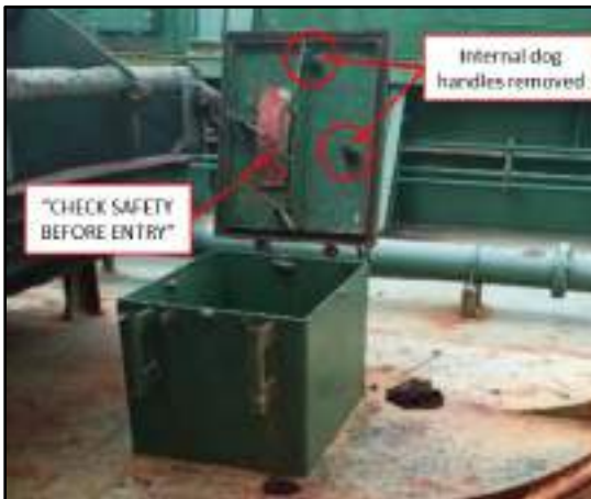
Figure 6 – The booby hatch cover for No.5 cargo hold (Source: The Company, annotated by the TSIB)
