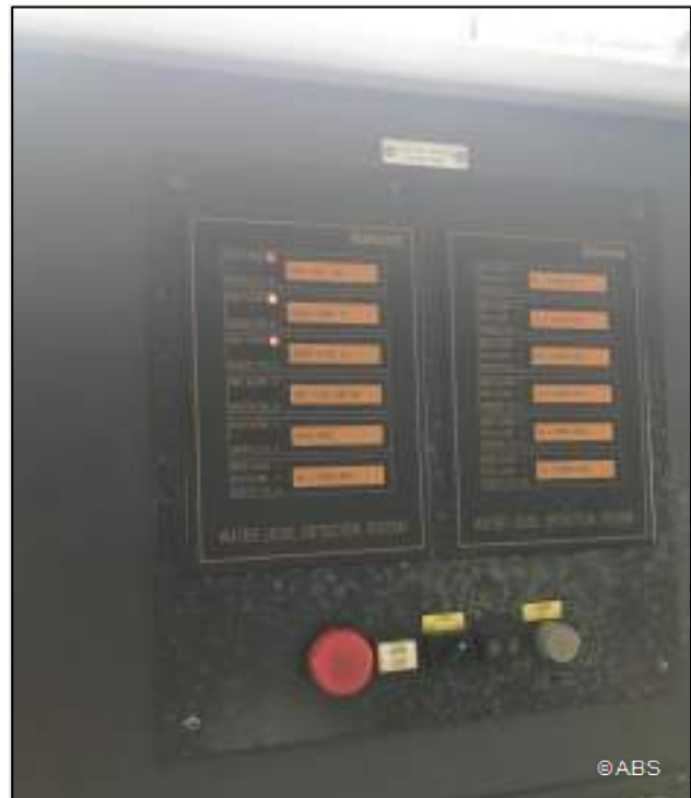
Water ingress alarm system defective
