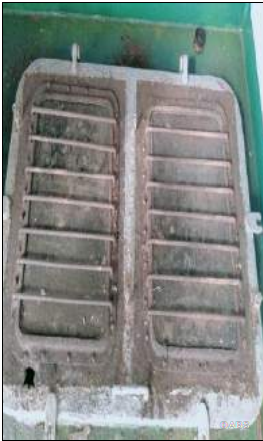
ER skylight door fitted with glass found excessively corroded with holes
