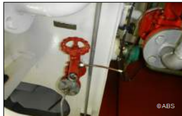
Quick closing valve for Emergency Diesel Generator supply was not available to close remotely
