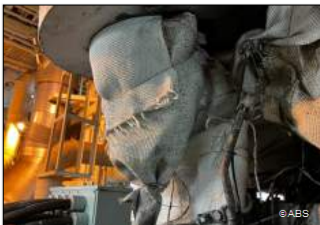
Diesel generator turbo charger insulation partly missing
