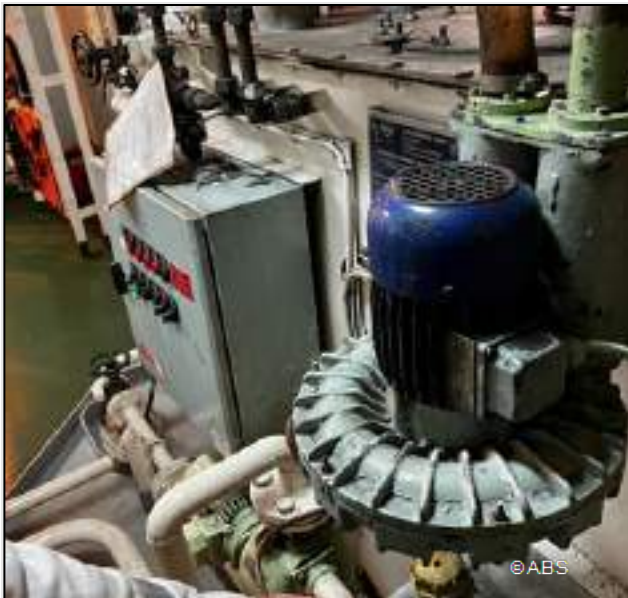
Sewage treatment plant not operable
