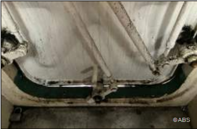
Accommodation weather tight door not able to fully close
