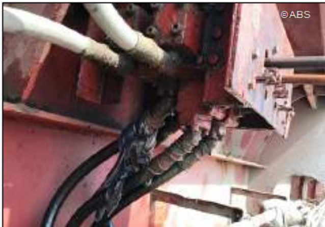
Cargo hold leaky hydraulic oil system
