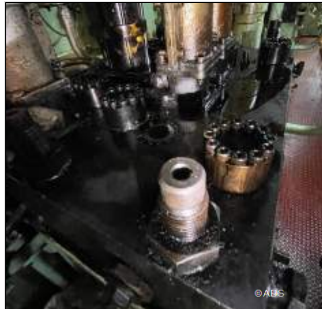
Fuel oil leakage from the ME fuel oil pump high pressure fuel line
