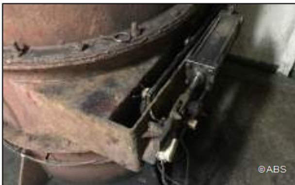
ER fire damper unable to operate (close)
