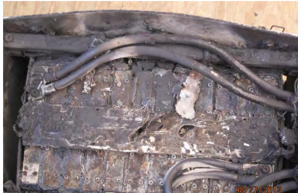
Burned out lithium-ion battery
