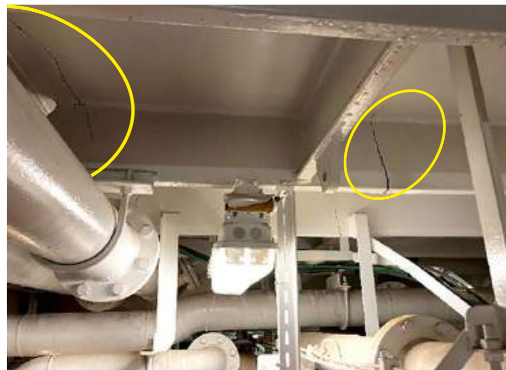
Figure 2: Cracks in the supporting steelwork
