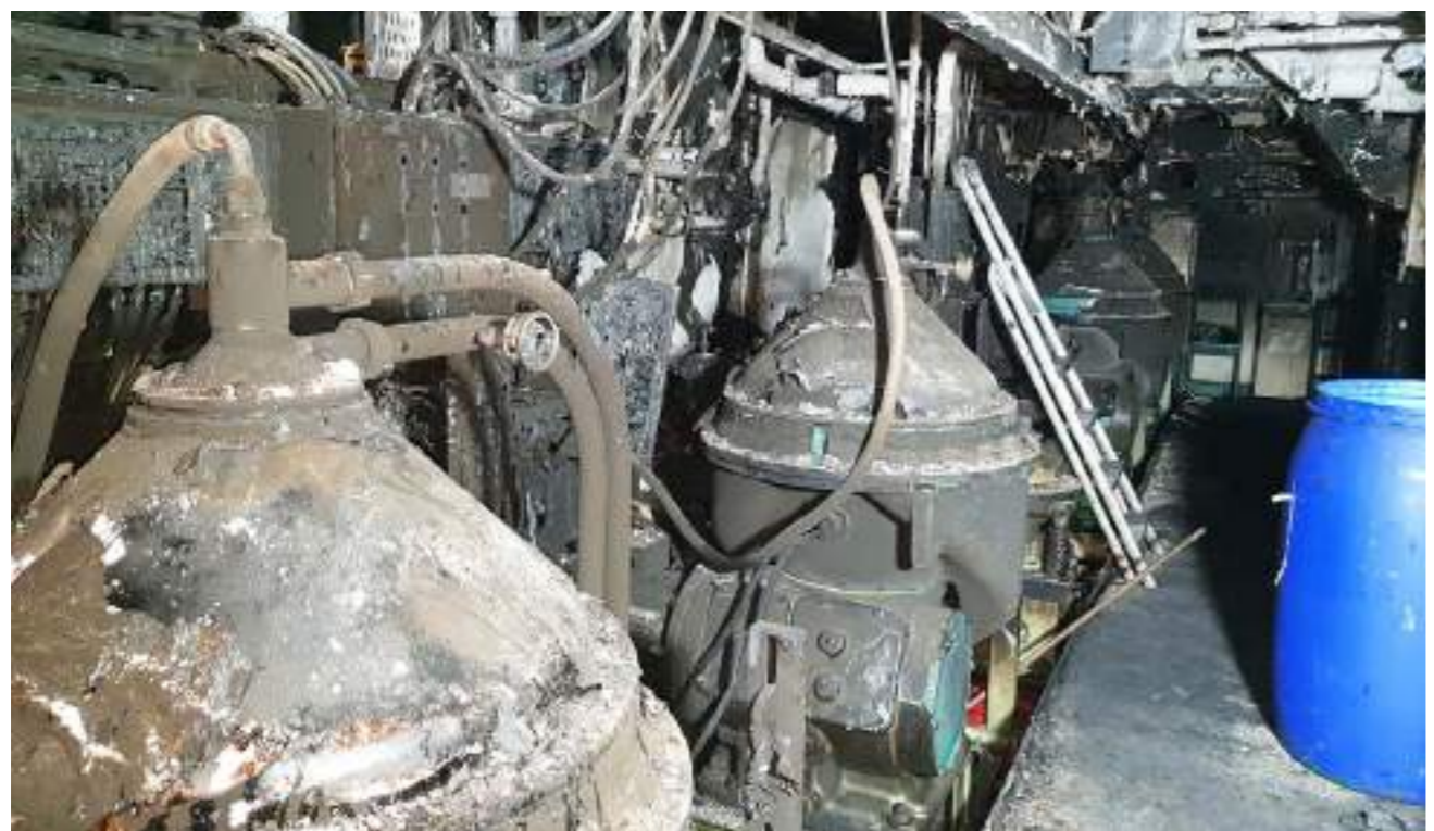
Figure 1: Fire-damaged fuel purifier room
