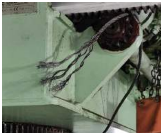
Figure 1: Failed crane hoisting wire
