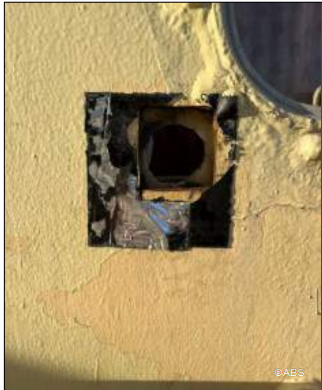
Unauthorized opening to accommodation bulkhead for fresh air access
