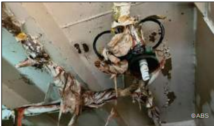
Insulation damage, electrical fixtures not maintained
