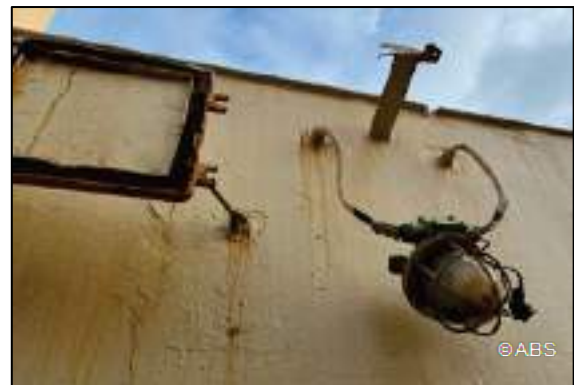
Deck fixtures are not maintained
