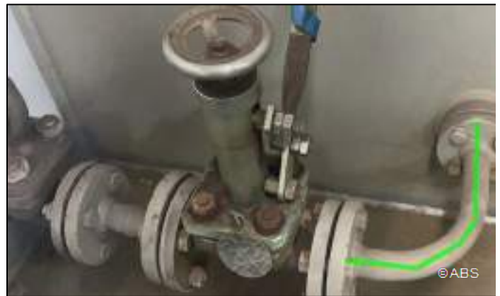
Emergency diesel generator quick closing valve fitted with 250mm apart from tank, does not meet requirement
