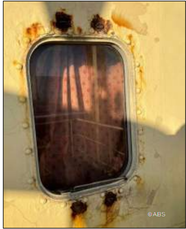
Safety bar missing from accommodation window
