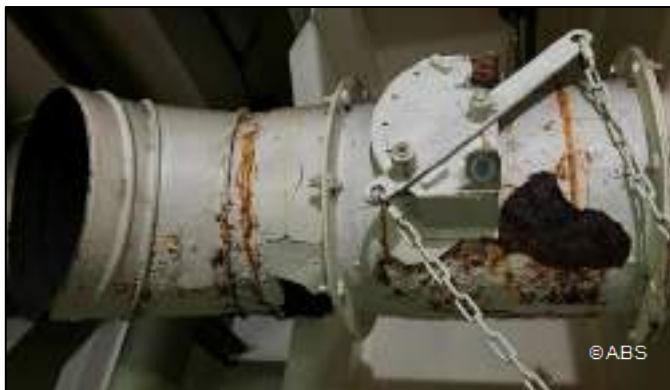
Wasted blower duct, inoperable flap
