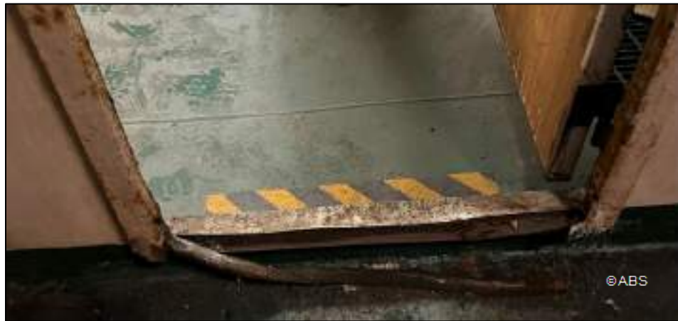
Fire door seal damage
