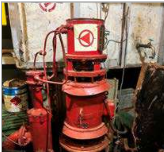
Emergency fire pump had water leakage from its coupling.
