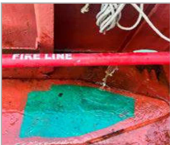
Fire line at STBD side adjacent to pilot station ruptured. [Not as required]
