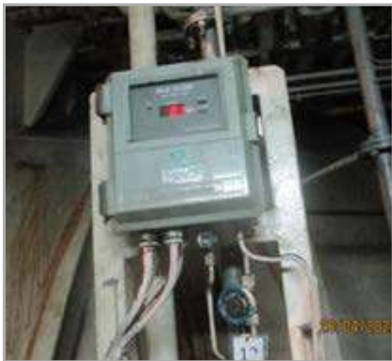
Oily water separator inoperative and not using for long time
