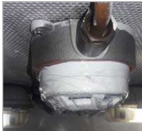
Fire detector in engine control room is covered by tape and not operational. [inoperative]
