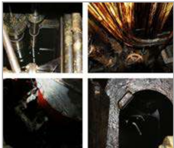
Several pipes (LT cooler / Main Sea water lines / fresh water lines) are leaking and temporarily repaired
