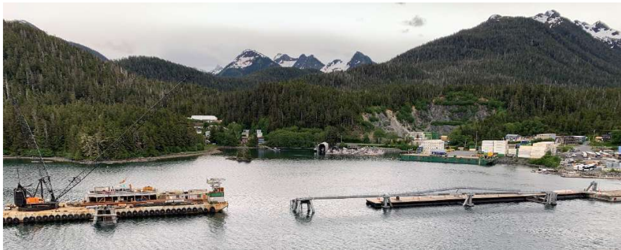
Figure 4. The Sitka Sound Cruise Terminal pier on June 9, 2022, with barge alongside the damaged dolphin for repairs (with catwalk between dolphins removed).
