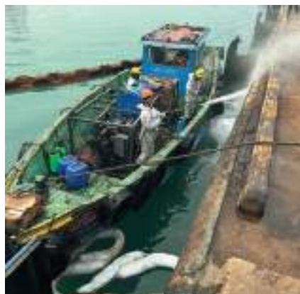
Cleaning port infrastructure, Thailand
