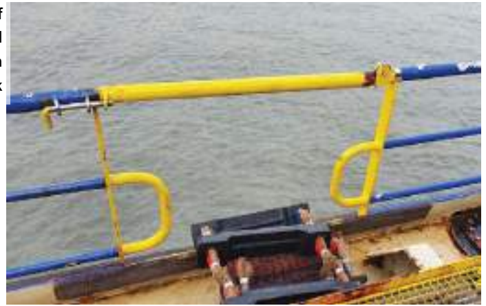
Figure 4: Second example of a noncompliant handhold stanchions for the transition from pilot ladder to deck
