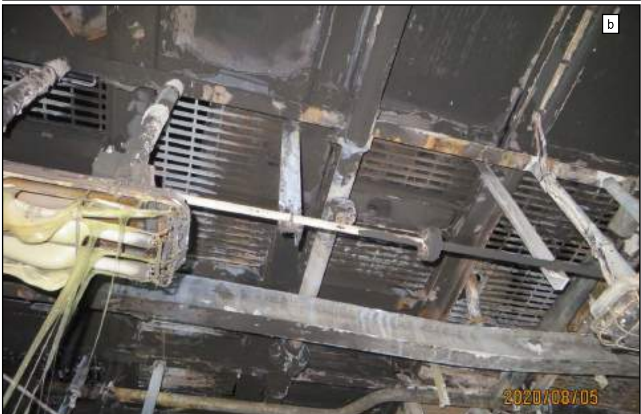
Figure 23: Boiler platform fire damage (a) and view up to boiler platform from auxiliary engines (b)
