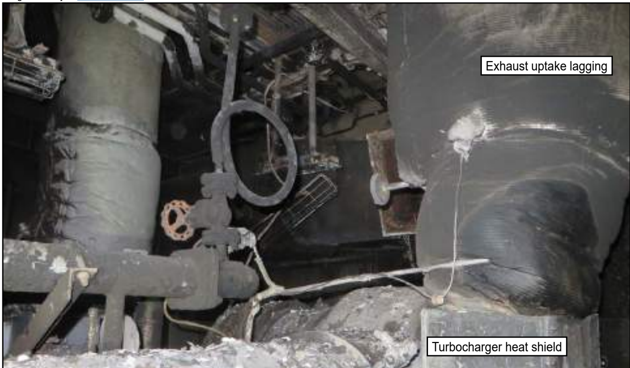
Figure 20: AE2 exhaust insulation
