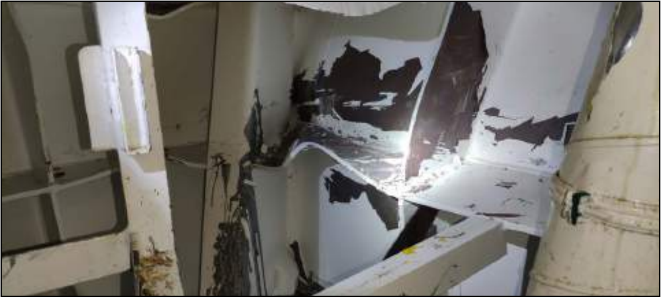
Figure 18: Damage to Scot Carrier 's internal bow structure
