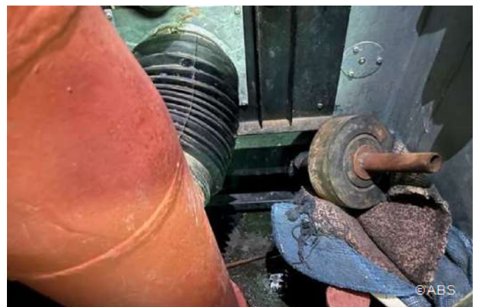
Sewage System Flexible pipe leaking
