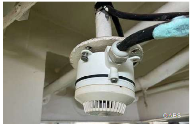
Fire detector not secured in the base
