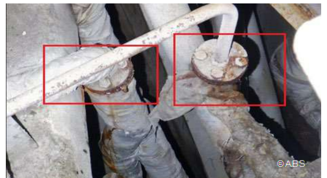
Steam pipe leaking
