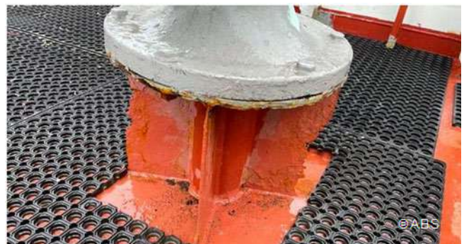
Bridge Wing Compass Pedestal wasted
