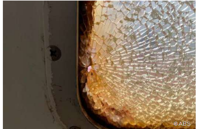
Accommodation window shattered with hole
