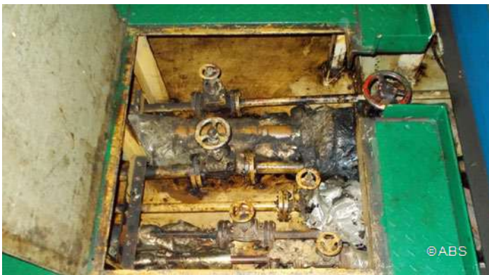
Purifier room fuel oil piping insulation missing
