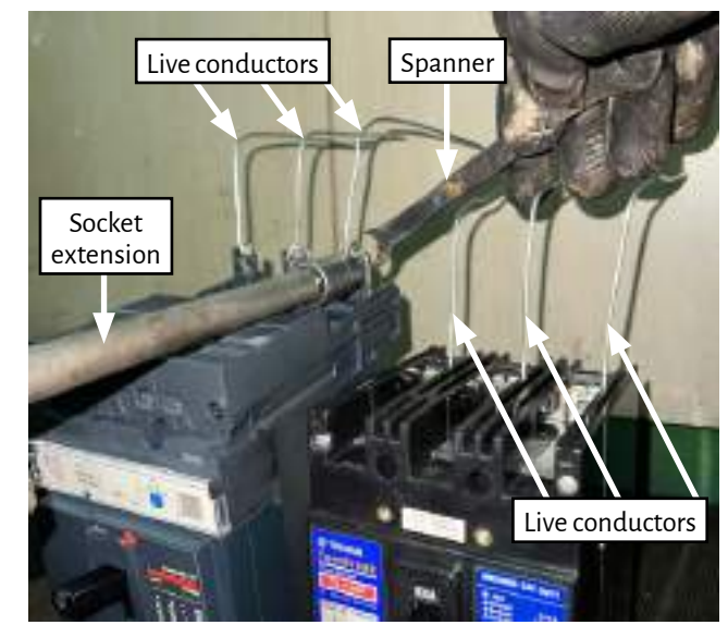
Figure 3: Reconstruction of the accident
