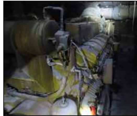
Figure 1: Damage sustained to auxiliary engine room
