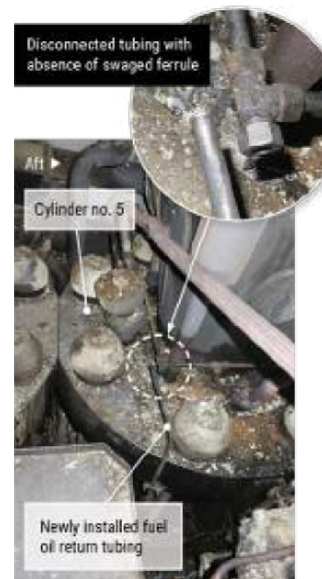
Figure 98. Cylinder no. 5 and the disconnected, newly installed fuel oil return tubing (inset).
