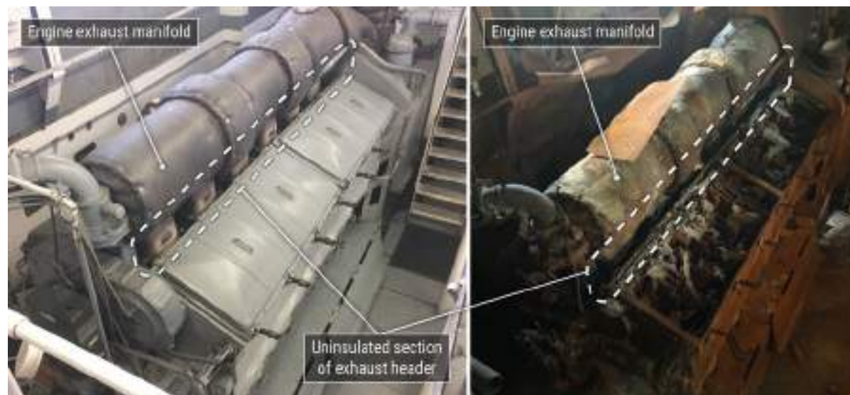
Figure 91. Starboard main engine before (left) and after (right) the fire, with the uninsulated section of exhaust header indicated. BACKGROUND SOURCE: WESTERN RIVERS BOAT MANAGEMENT INC.
