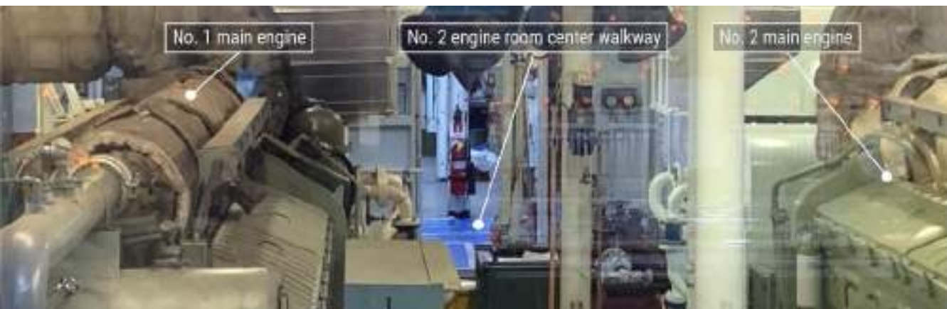
Figure 140. No. 1 engine room diesel engines as seen from the engineering operating station; center walkway of the no. 2 engine room is through the open door in the background. SOURCE: WASHINGTON STATE FERRIES
