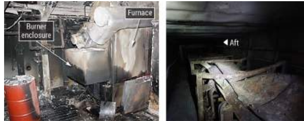
Figure 104. Left to right: Fire-damaged furnace and conveyor belt within the conveyor belt trunk above the furnace. SOURCE: COAST GUARD
