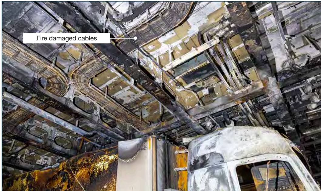
Figure 36: Fire damages to the deck head above the burning truck. Source: DMAIB
