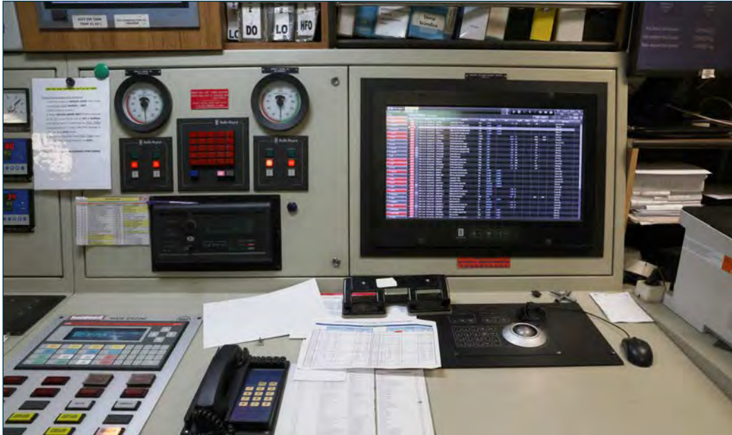
Figure 44: Monitor for alarm monitoring system. Source: DMAIB
