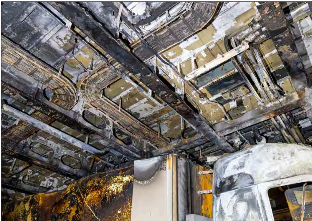
Figure 42: Burnt cable trays visible directly above the truck. Source: DMAIB
