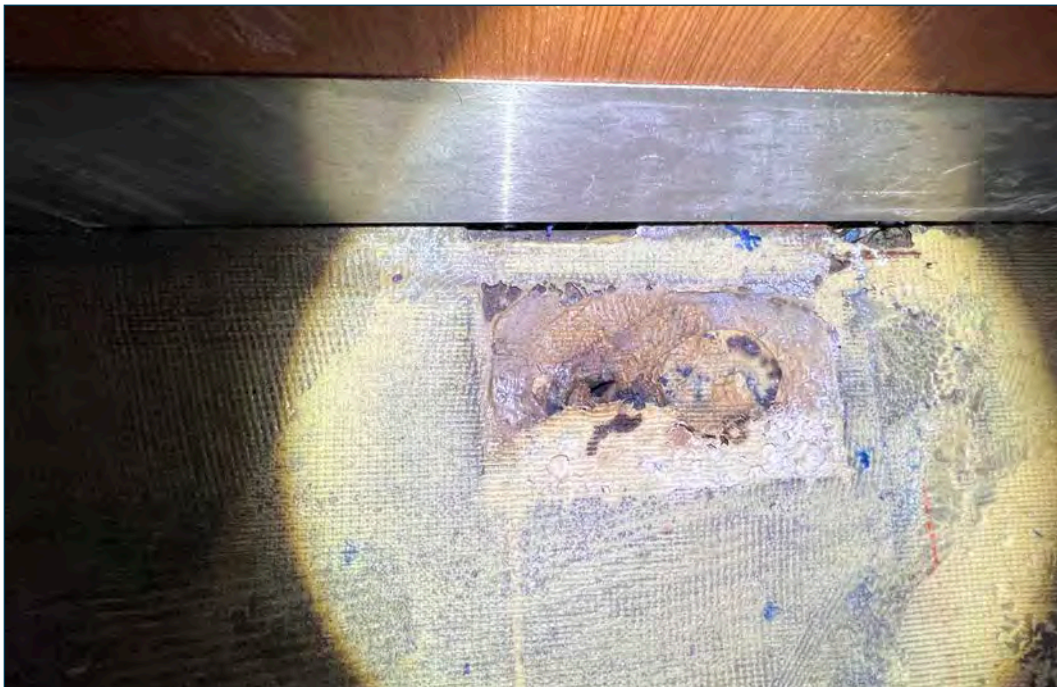
Figure 38: Heat damage to the adhesive. Source: DMAIB
