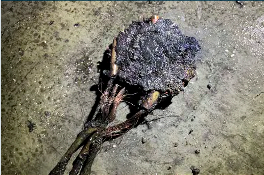
Figure 21: Melted power cable inlet. Source: DMAIB
