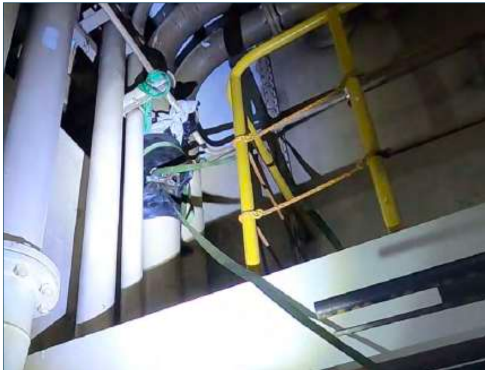
Figure 9: Sealed off drencher pipe leakage. Source: DMAIB
